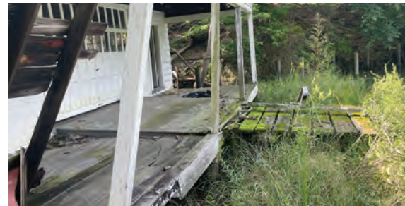
Existing Boathouse Platform: The deteriorated boathouse structure will be stabilized and repurposed as an elevated scenic overlook, providing passive educational opportunities and expansive views of Loden Pond and the South River.
