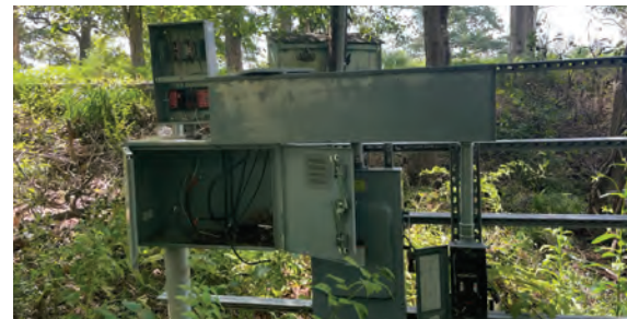
Existing Electrical Panel Near Boathouse: Abandoned electrical infrastructure associated with the former boathouse, slated for removal as part of shoreline restoration and safety improvements.
