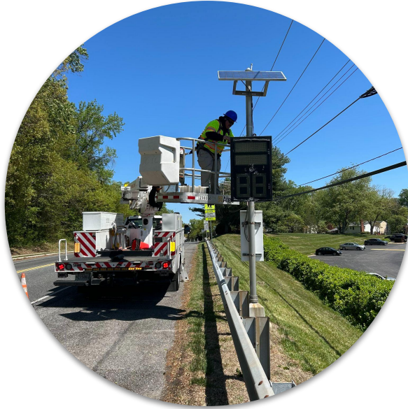
Traffic Signal Asset Maintenance
