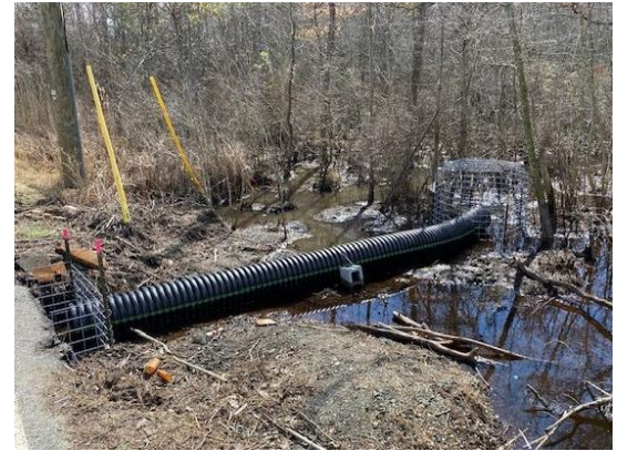
Culvert protection device
