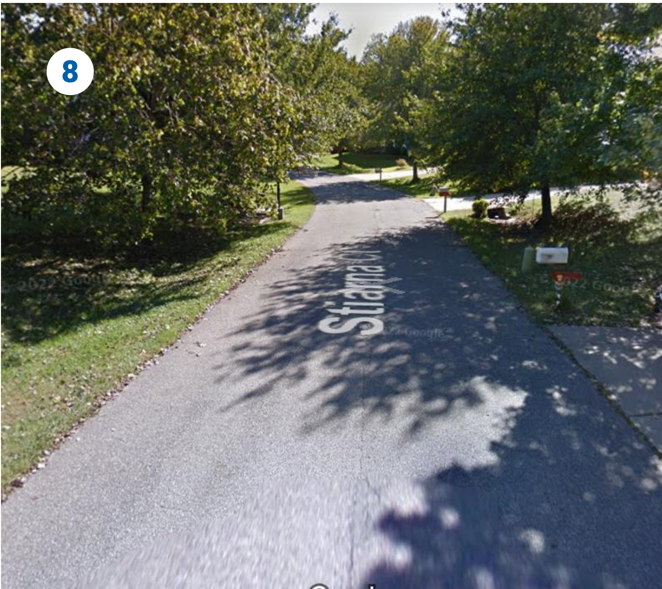
Stiarna Court – missing sidewalk
