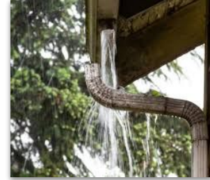
Disconnected Roof Gutter
