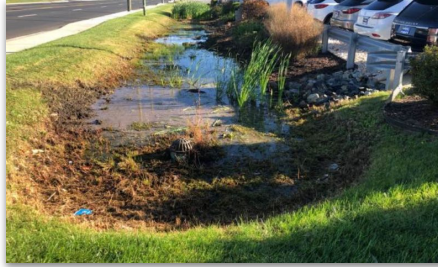
Standing Water (Blocked Underdrain)
