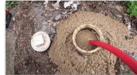
Blocked Underdrain, Cleanout, Observation Well
