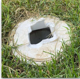
Broken, Buried, or Missing Cleanout/Observation Well Caps
