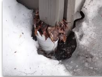
Clogged Downspouts, Disconnection from Ground Connector
