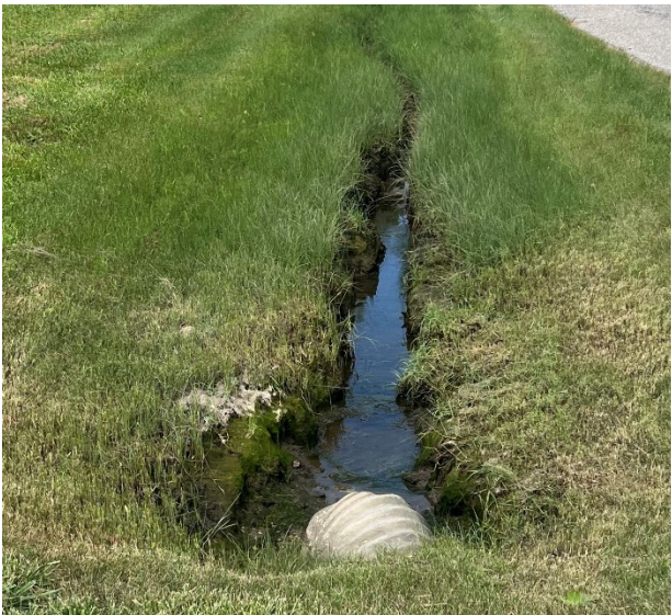
Photo 49 - Standing water in driveway culvert/swale system
