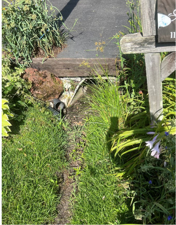
Photo 48 - Sedimentation in driveway culvert
