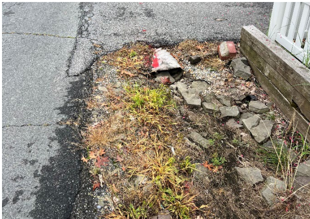
Photo 107 - Crushed driveway culvert
