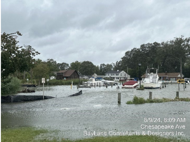
Photo 42 - Marina bulkhead completely overtopped, and some areas flooded more than two feet Water level: +3.77' NAVD88 (or 3.11' above MHW)
