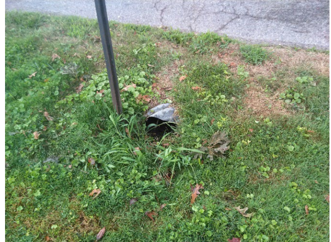
Photo 87 - Overgrown roadway culvert
