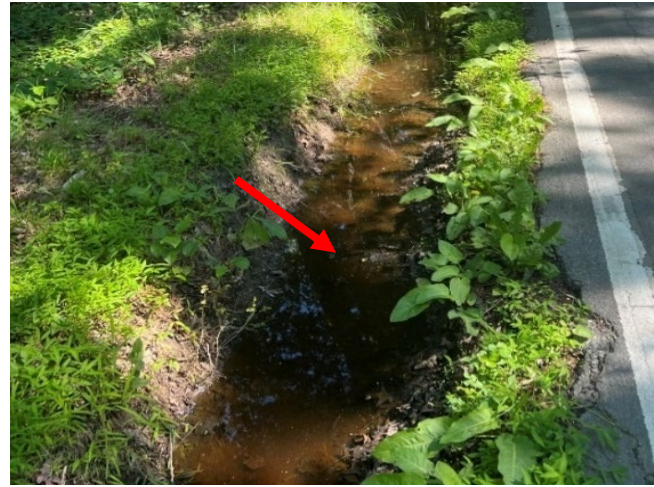
Photo 30 - Pooling water in roadside swale with damage to edge of pavement
