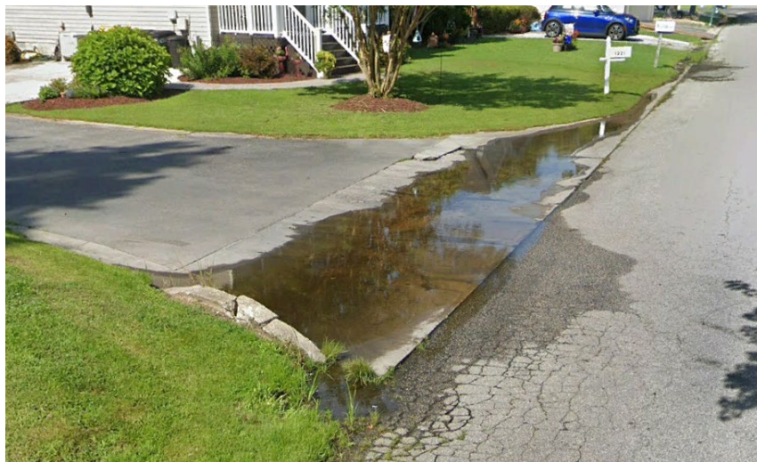
Photo 24 – Standing water and road damage at Johnson Drive and Magnolia Ridge Road intersection
