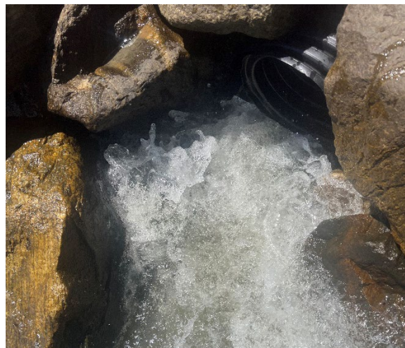
Photo 31 - Tidal outfall without backflow prevention Water level: +0.38' NAVD88 (or .28' below MHW)
