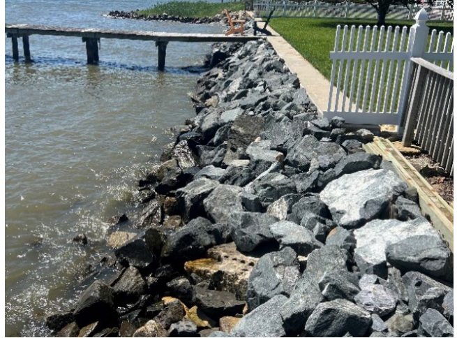
Photo 26 - Timber bulkhead and seawall with stone protection (Top of Wall and Stone +5' NAVD88)
