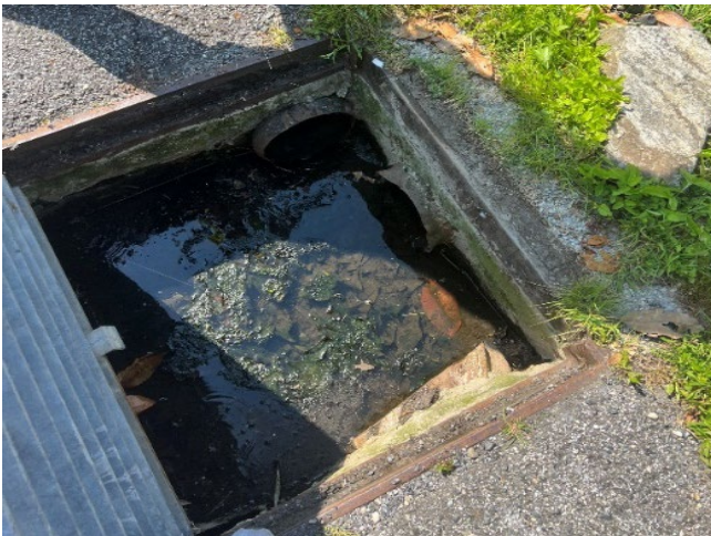
Photo 40 - Inlet blocked by sediment and debris
