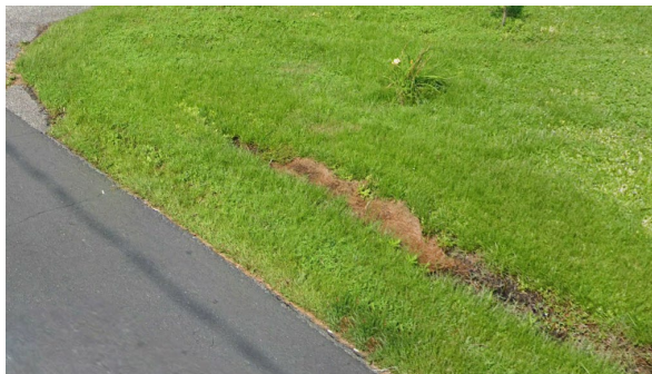
Photo 19 - Sedimentation blocking proper conveyance through road culvert
