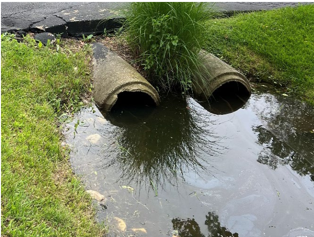
Photo 13 - Driveway culvert and swale backwatered at high tide Water level: +2.16' NAVD88 (or 1.5' above MHW)
