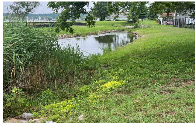
Photo 112 – Backwatering at gap in seawall at 6089 Melbourne Avenue. Water level: +1.14' NAVD88 (or 0.48' above MHW)
