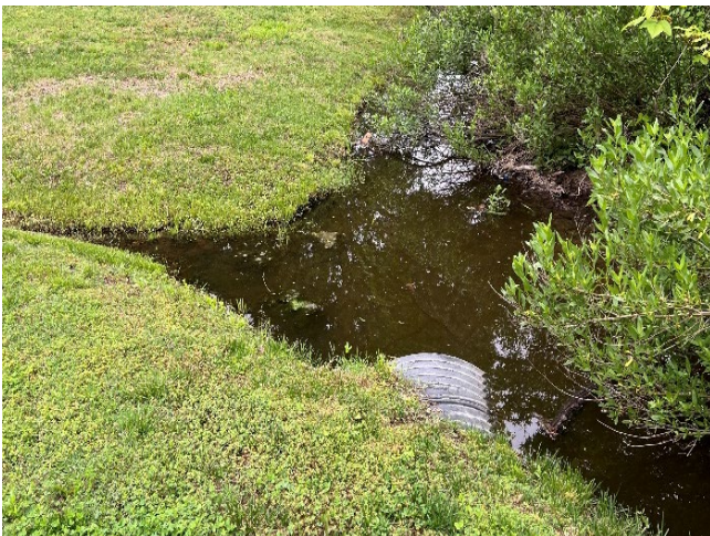
Photo 11 - Outfall almost completely submerged at high tide Water level: +1.73' NAVD88 (or 1.07' above MHW)
