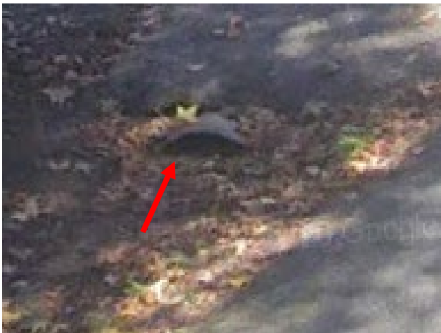
Photo 67 - Sedimentation blocking stormwater conveyance through driveway culvert and swale system
