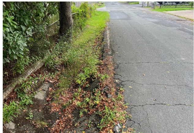
Photo 108 - Overgrowth and sedimentation in roadside swale
