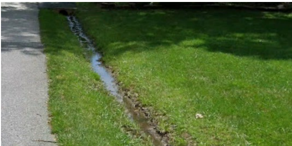
Photo 93 - Pooling water and sedimentation in grassy swale at the intersection of 1st Street and Main Street.
