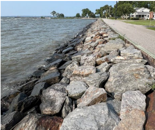
Photo 73 - Seawall fronted by revetment along Chesapeake Drive (Top of Bulkhead +6.5' NAVD88; Top of Stone +6.0' NAVD88)
