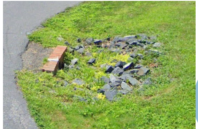
Photo 84 – Roadway culvert blocked by stone and overgrown vegetation
