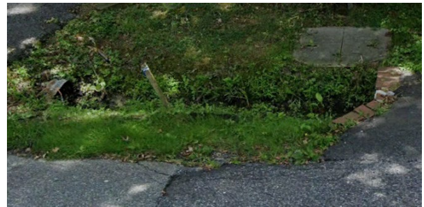
Photo 94 - Series of driveway culverts connected by overgrown grassy swale.
