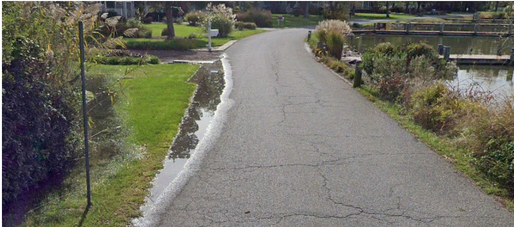
Photo 66 - Standing water on road edges
