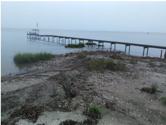
Photo 88 - Degrading natural shoreline due to increased exposure at remnant island is submerged.
