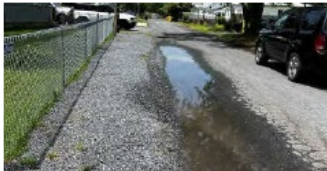
Photo 61 - Water ponding due to swale removal
