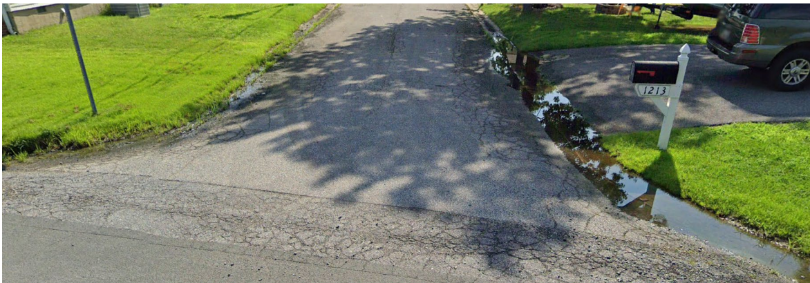
Photo 23 – Road damage due to standing water on pavement at Johnson Drive and Olive Street intersection
