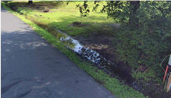
Photo 21 - Pooling in roadside swale along Lee Boulevard
