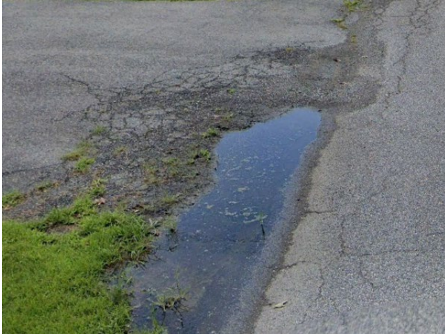
Photo 86 - Standing water leads to roadway degradation.
