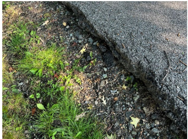
Photo 41 – Eroding edge of pavement
