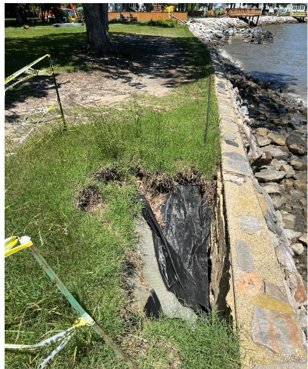
Photo 28 - Washout behind seawall
