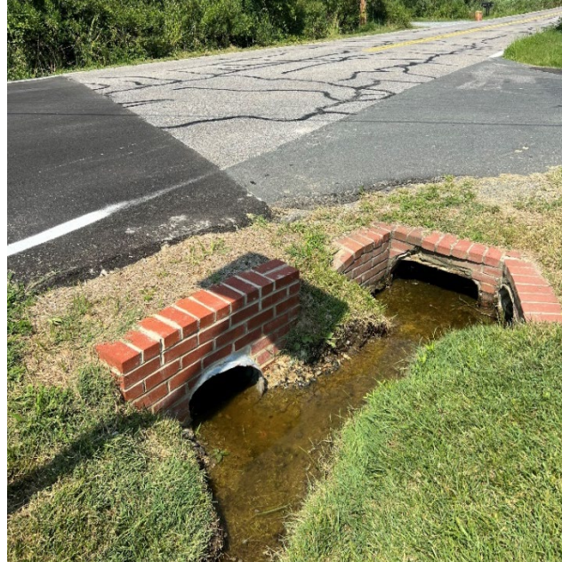
Photo 81 - Backwatering of roadway culverts at the intersection of Gwynne Avenue and Dartmouth Street; road repairs along Gwynne Avenue indicating damage due to frequent flooding.
