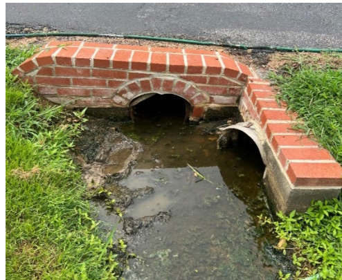
Photo 110 – Roadway culverts connecting conveyance systems across Owings Beach Road to outfall into adjacent wetland (Invert Elevations +1' to +1.4' NAVD88) Water level: +0.72' NAVD88 (or 0.06' above MHW)
