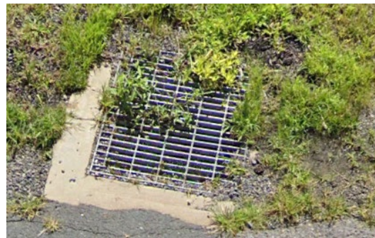
Photo 20 - Overgrown storm grate
