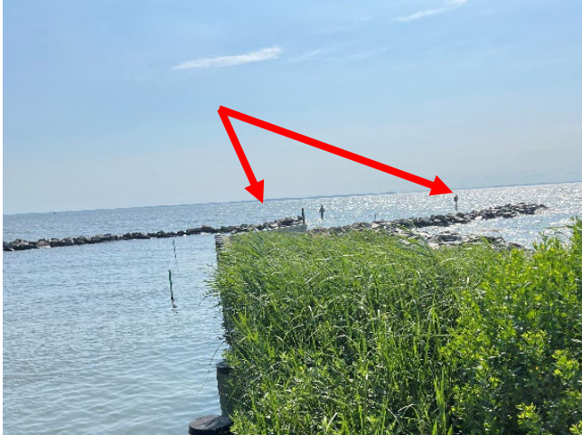
Photo 32 - Stone jetties at Snug Harbor basin entrance (Top of Stone +2.0' to +3.0' NAVD88)
