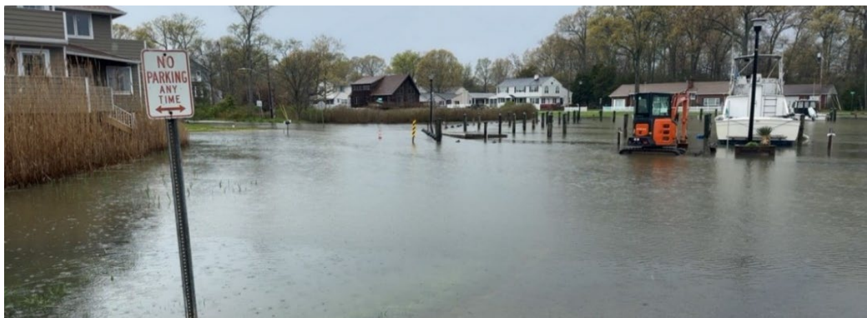
Photo 46 - Cedarhurst Marina bulkhead overtopped during high tide event (April 12, 2024) Water level: +2.71' NAVD88 (or 2.05' above MHW)
