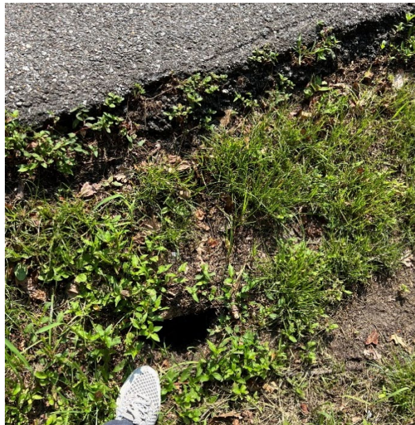
Photo 79 - Culvert blocked by sedimentation and overgrowth; road edge erosion
