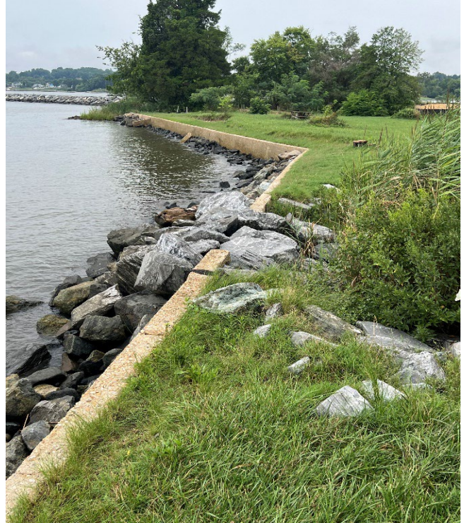
Photo 103 - Gap in seawall at southernmost property in Owings Beach
