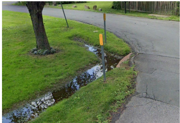
Photo 100 - Roadway culvert that outfalls to tidally influenced marsh area is backwatered into connecting swale system
