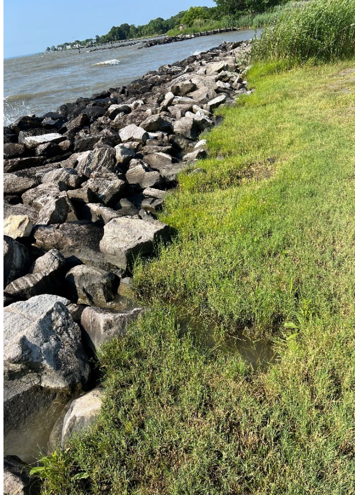
Photo 35 – Undermining of stone protection along Snug Harbor's shoreline with direct bay exposure
