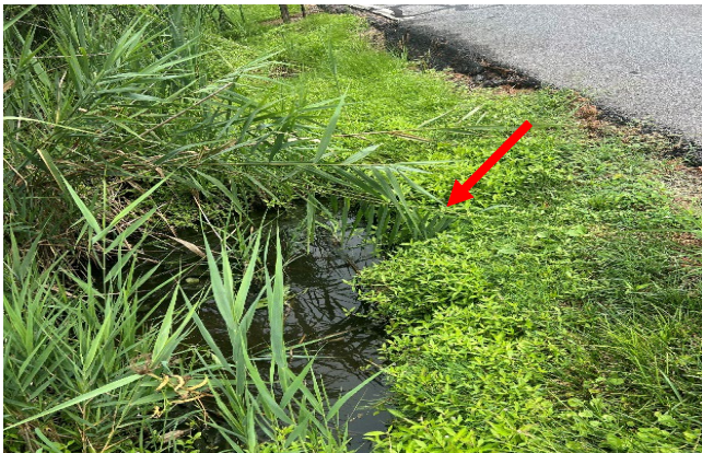
Photo 111 – Submerged and overgrown outfalls (Invert Elevations +0.36' to +0.58' NAVD88) at Owings Beach Road Water level: +0.74' NAVD88 (or 0.08' above MHW)
