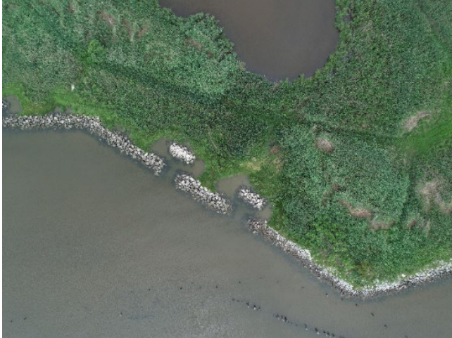
Photo 97 - Stone protection at edge of marsh along bay-facing shoreline (Marsh interior +1.0 - +3.0 feet NAVD88; Top of Stone +1.5 feet NAVD88)
