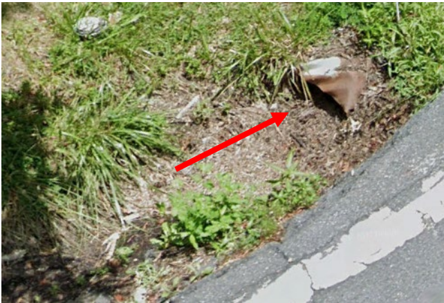
Photo 83 - Partially blocked driveway culvert on Battee Drive
