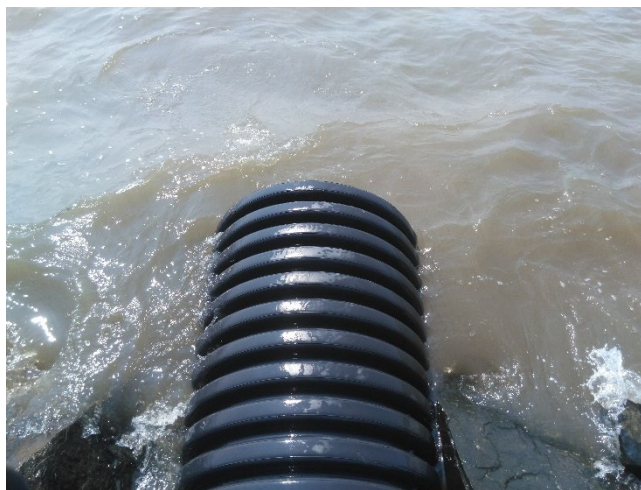
Photo 82 - Tidal outfall partially inundated along Chesapeake Drive Water level: +1.52' NAVD88 (or 0.8' above MHW)
