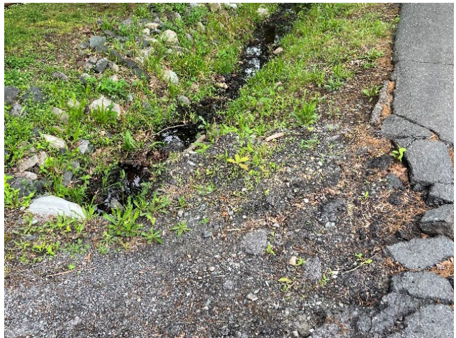
Photo 14 - Swale and culvert with standing water and road damage
