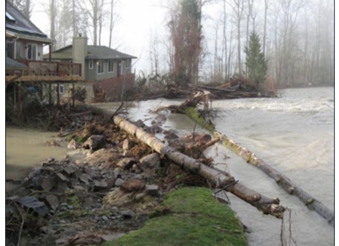
Photo 136 - Lower Snoqualmie Basin Levee Breach in 2009 – Photo by King County
