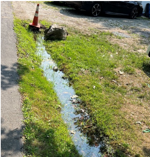
Photo 78 - Standing water in roadside swale due to crushed driveway culvert
