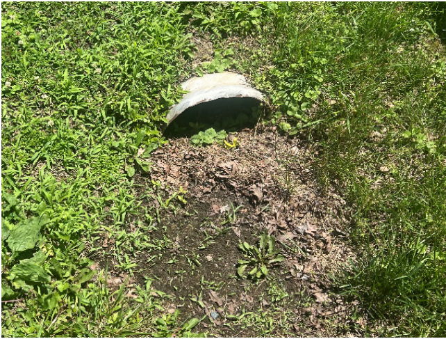
Photo 29 - Sedimentation blocking driveway culvert
