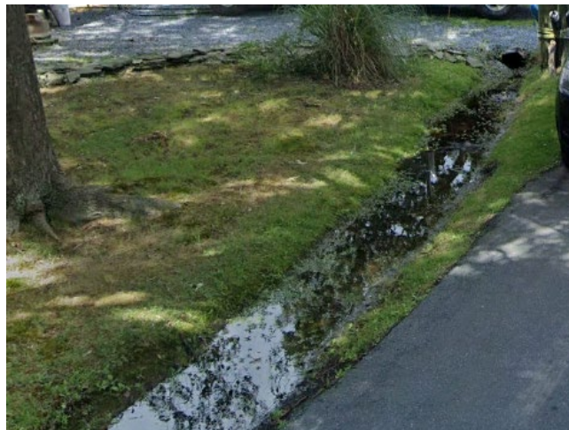
Photo 85 - Standing water in grassy swale along Bay View Parkway
