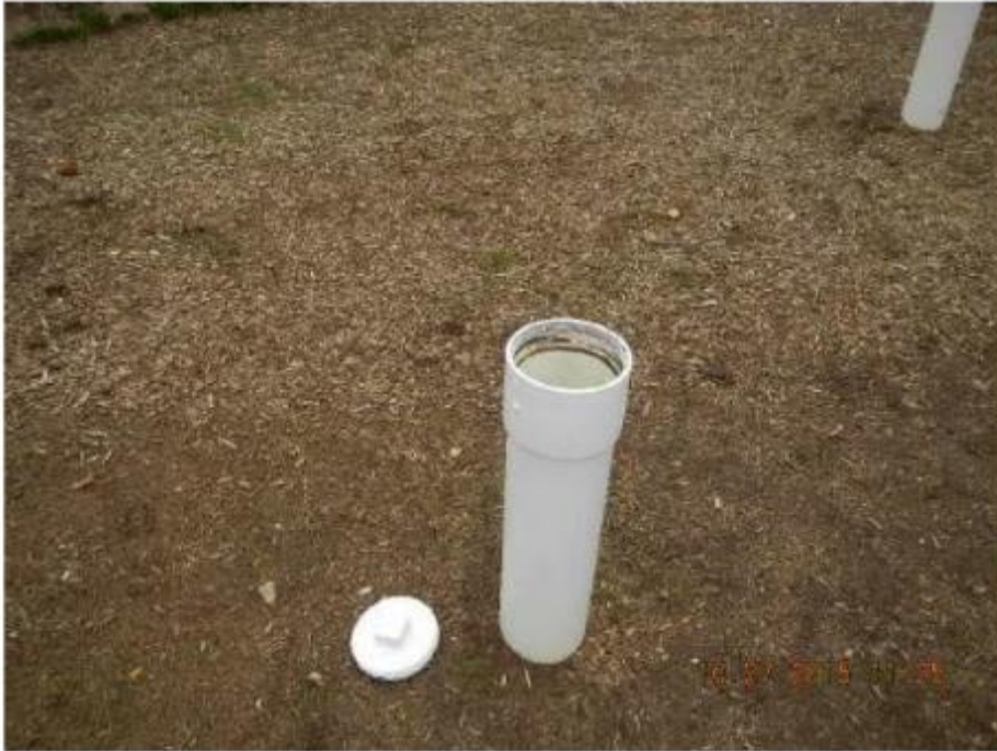
A typical cleanout, extending higher than 12 in. above the ground surface.
