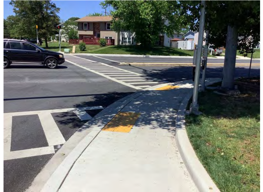
After - to meet regulatory requirements
