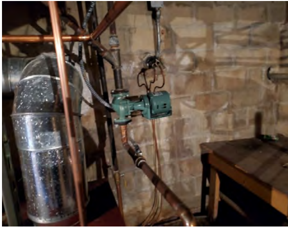
Hot Water Boiler Pump
