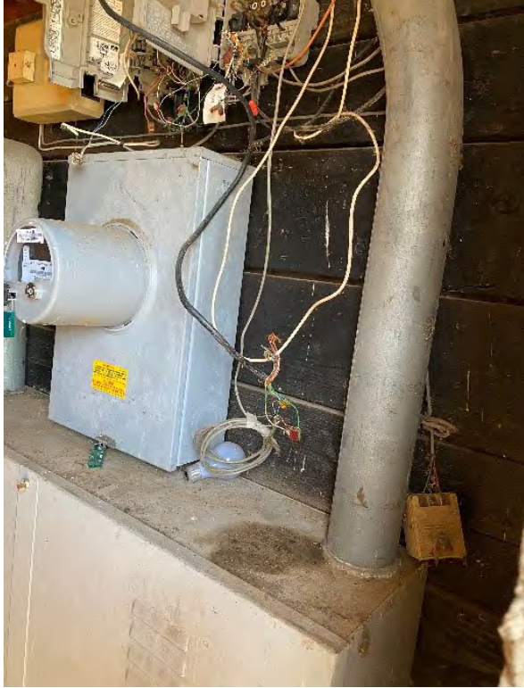
Room 411 - Abandoned Cabling
