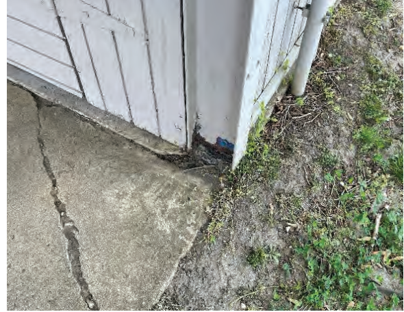
View of column base requiring repair and stabilization from ongoing deterioration.
