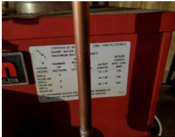
Hot Water Boiler
