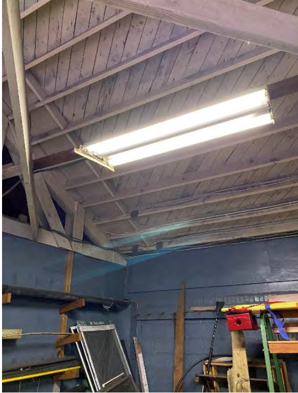
Room 402 - Typical Light Fixture
