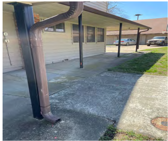
8.4.2 Example of downspout discharge.
