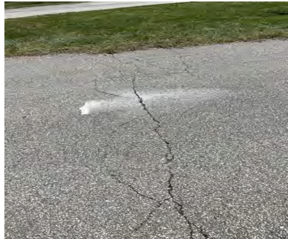
8.1.2 Alligator cracking in pavement.
