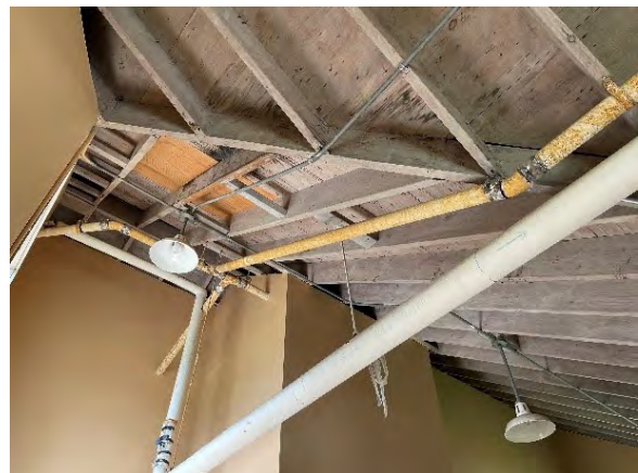
Interior view of the valley with replaced sheathing, Located on the Women's side.
