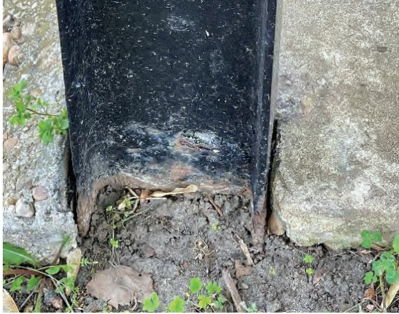
Column base detail with corrosion, Base condition to be repaired.
