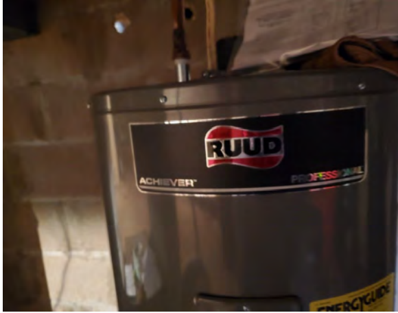
Domestic Water Heater
