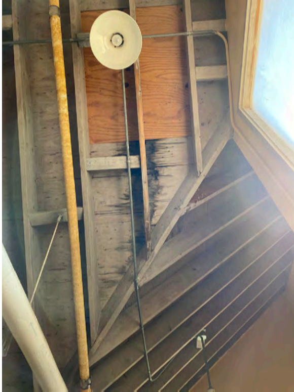
Interior View of Wood Rafters and Leak Stain
