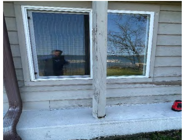
View of twisted column and concrete wash repair.
