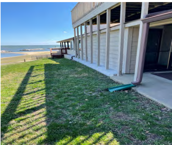
8.4.3 Example of downspout discharge.
