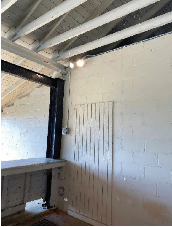
Typical Exterior Lighting
