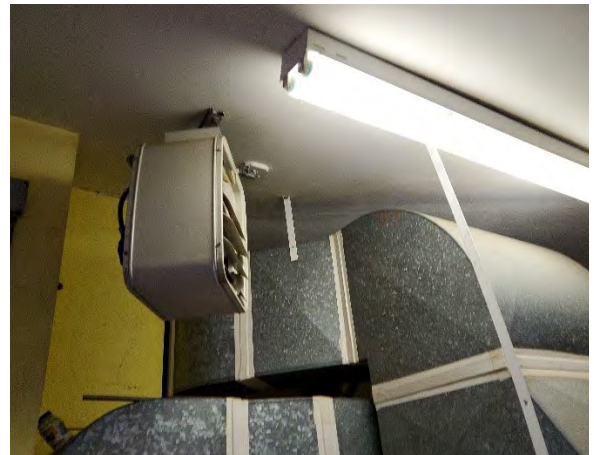
Mechanical Unit Heater
