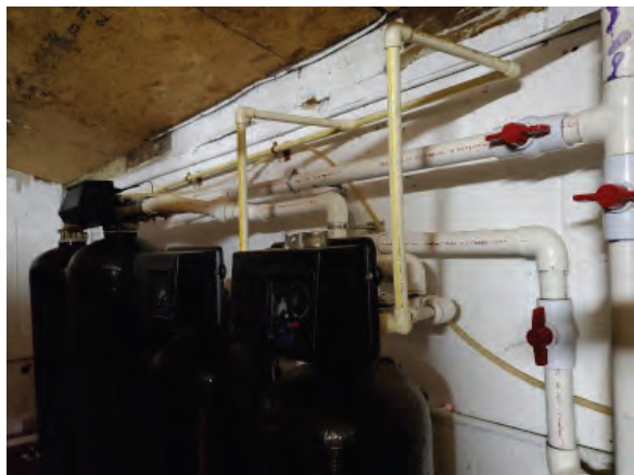
Campus Water Filtration System
