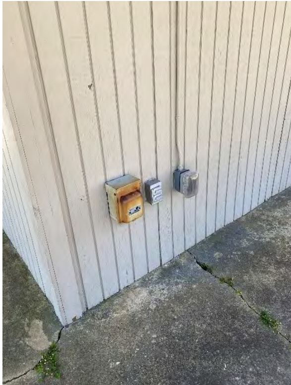
Disconnect and Outdoor Receptacles
