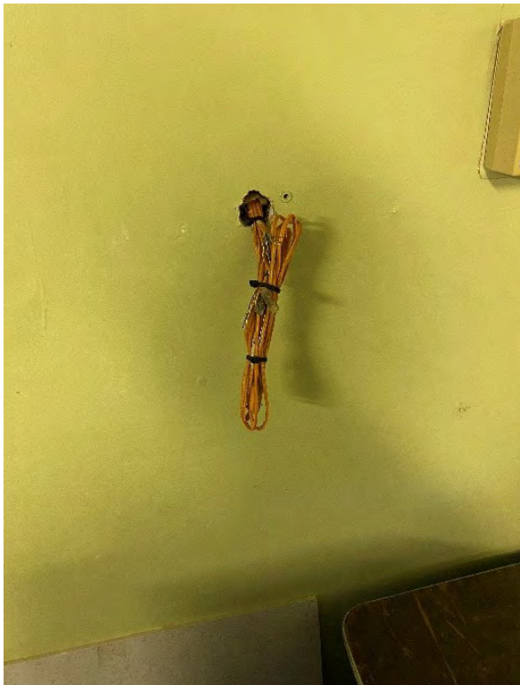
Abandoned Cabling (Typical)
