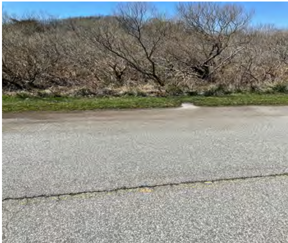
8.1.1 Cracked asphalt pavement at entrance road.
