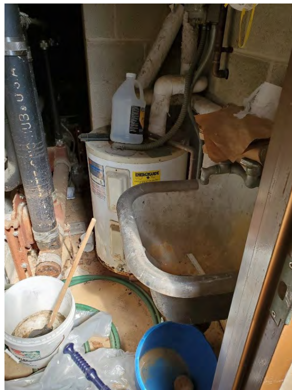
Domestic Water Heater
