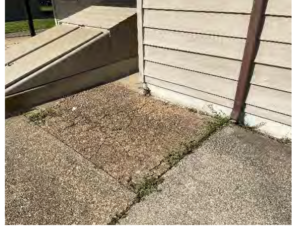
View of settled exterior concrete slab.
