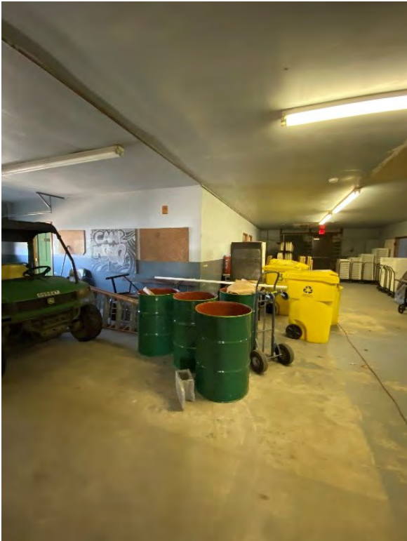
Room 401 - Typical Light Fixtures
