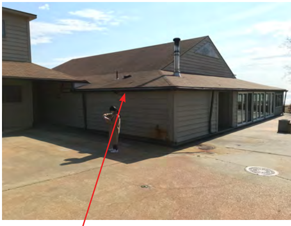
Damaged gutter and downspout
