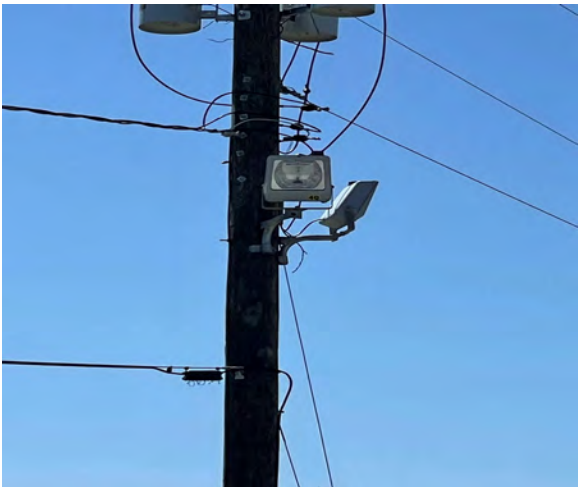
8.6.3 Existing site lighting on BGE pole.
