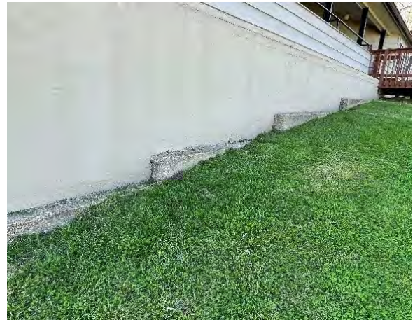
Stepped footing exposed, suspect not below frost line
