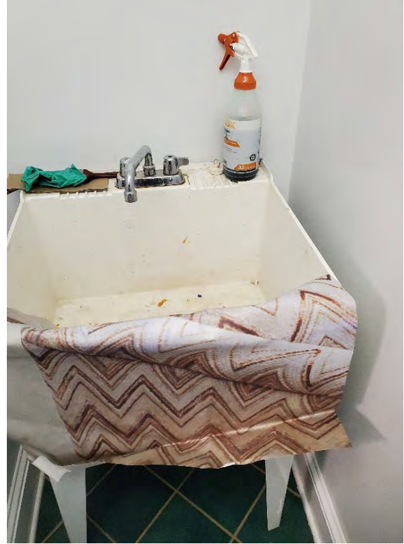
First Floor Laundry Sink
