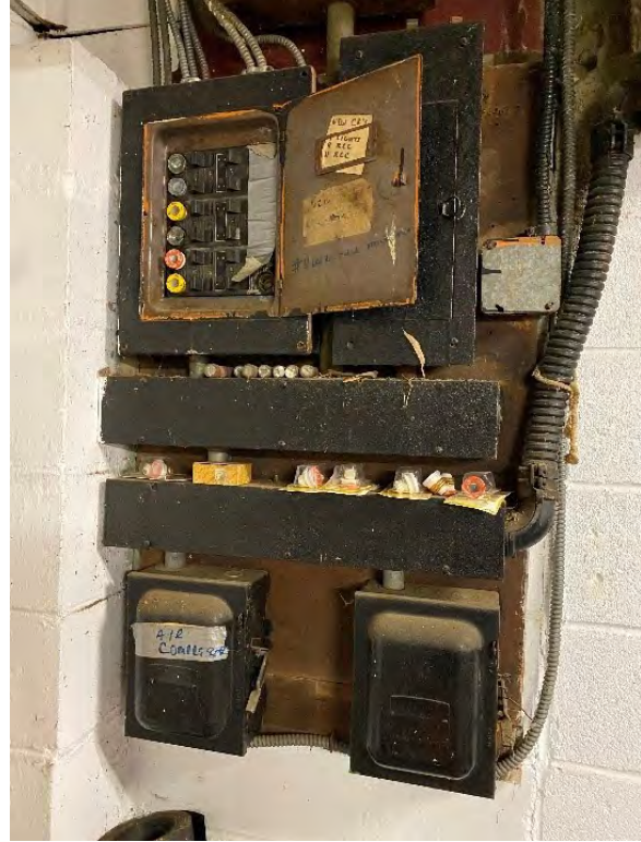
Room 412 - Aged Electrical Equipment
