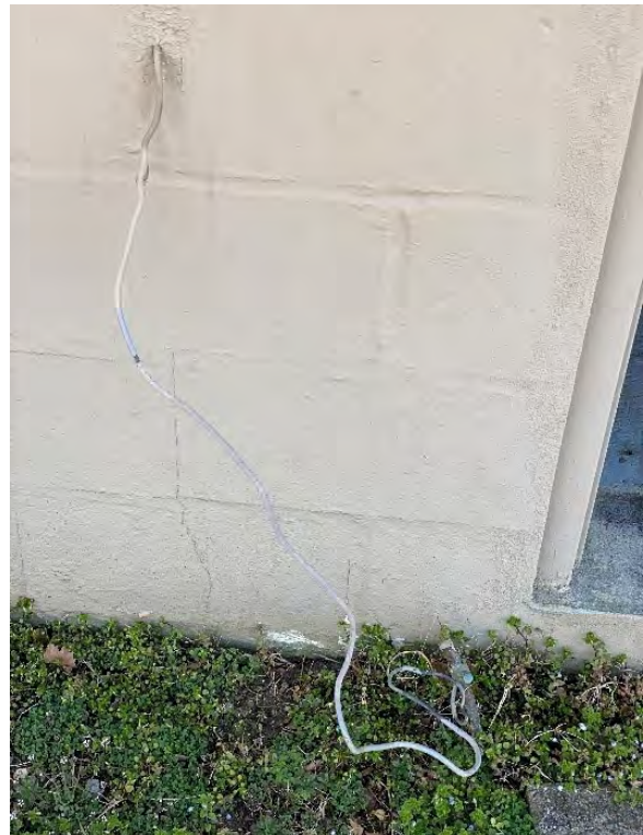
Building Grounding System
