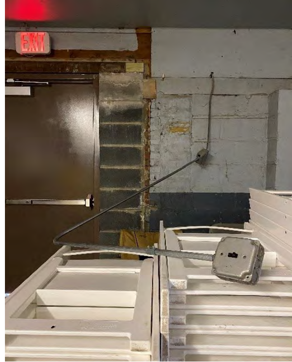
Room 401 - Light Switch Mounting
