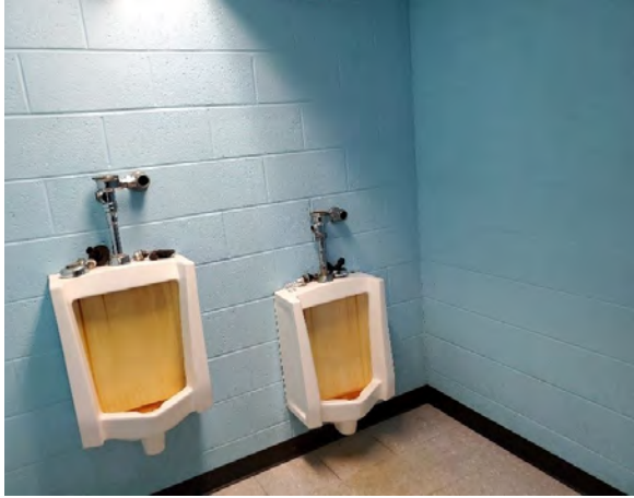
Men's Bathroom Urinal
