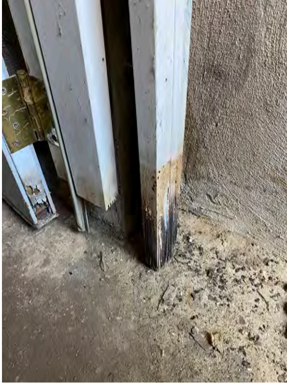
Door & frame damage at 201/B
