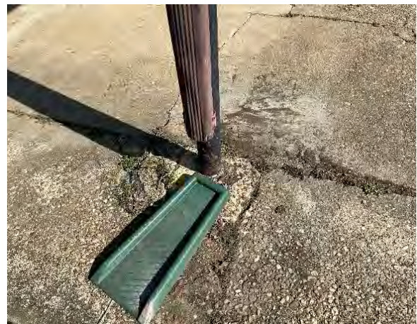
Steel column base with deteriorated concrete and missing downspout extension.
