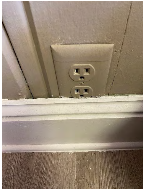
Receptacle in Floor Molding
