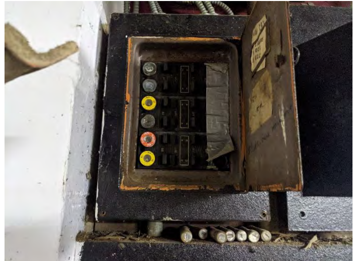
Breaker box with empty fuse opening covered with tape
