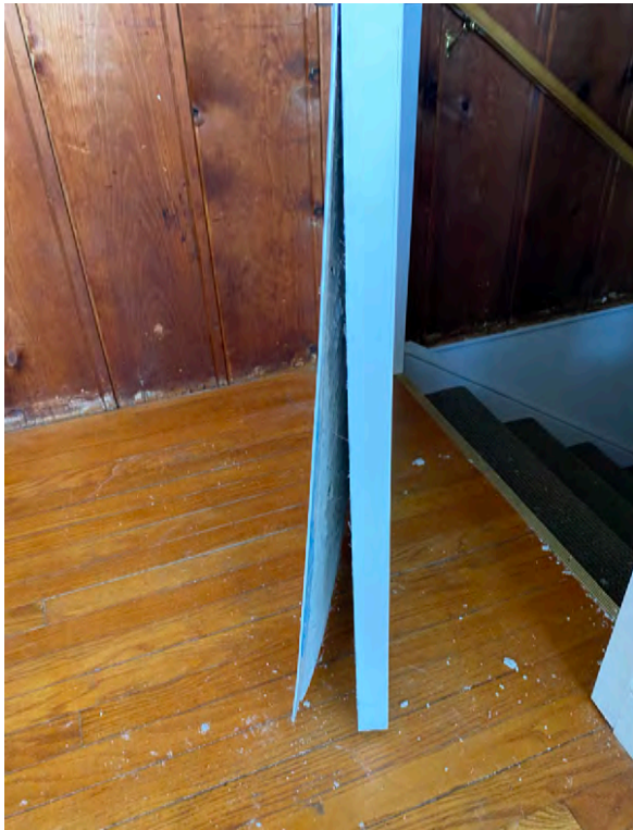
Door damage at 208/E
