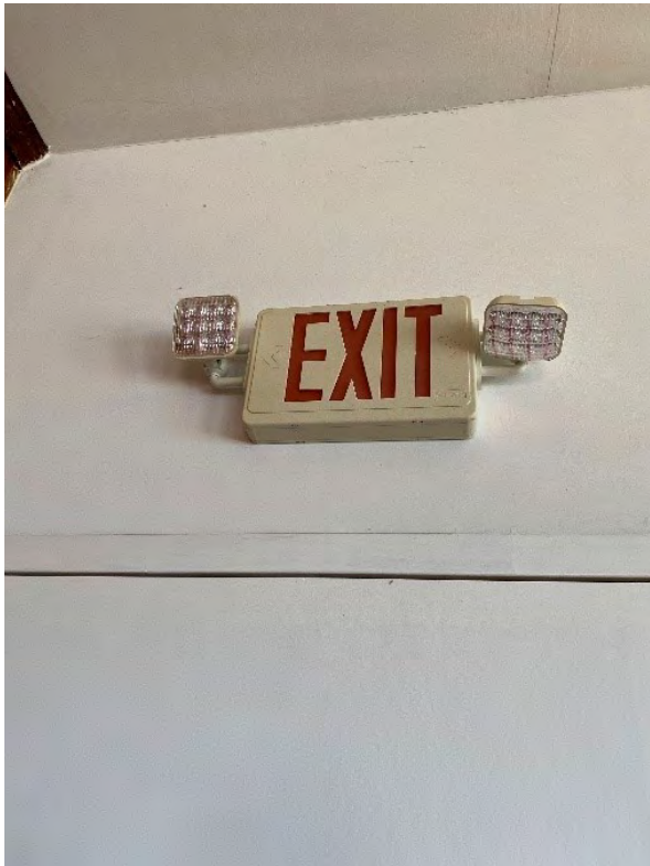
2nd Floor Exit Sign not Illuminated
