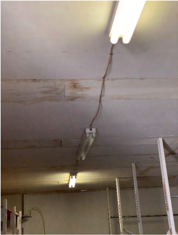
Non-working Lighting Fixture
