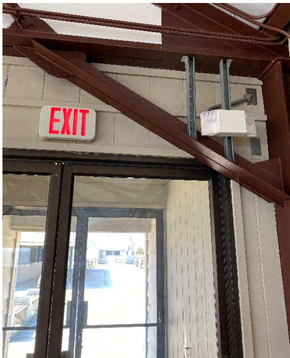
Typical Emergency Wall Pack
