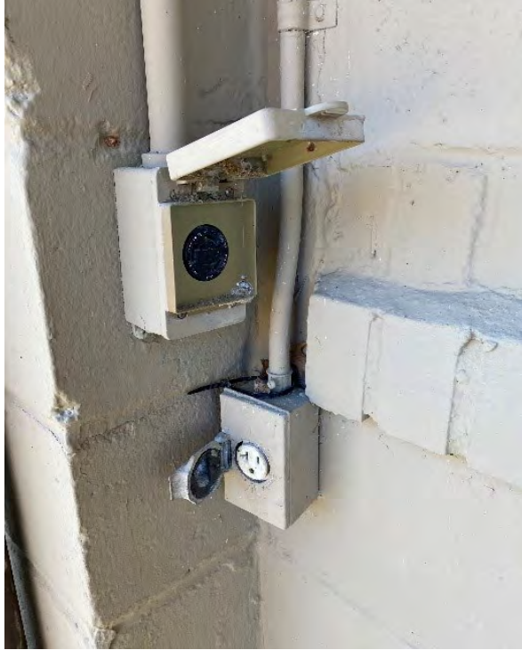
Outdoor Non-GFCI Receptacles
