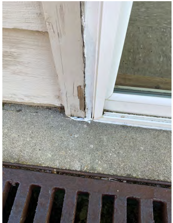
Deteriorating siding and trim
