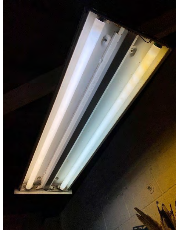
Room 407 - Typical Light Fixture
