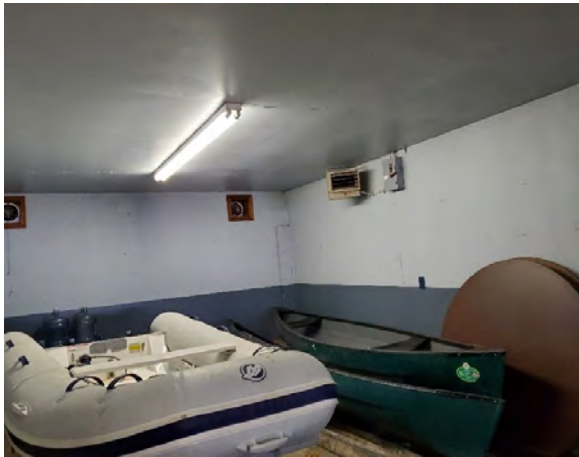
Electric Unit Heater and Exhaust Fan in Storage Area
