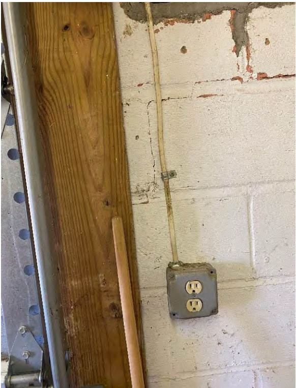
Typical Indoor Wiring
