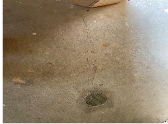
View of minor shrinkage cracking in floor slab.
