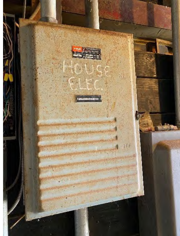
Room 411 - Typical Disconnect
