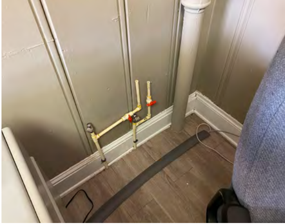
Office 202 - Exposed water lines
