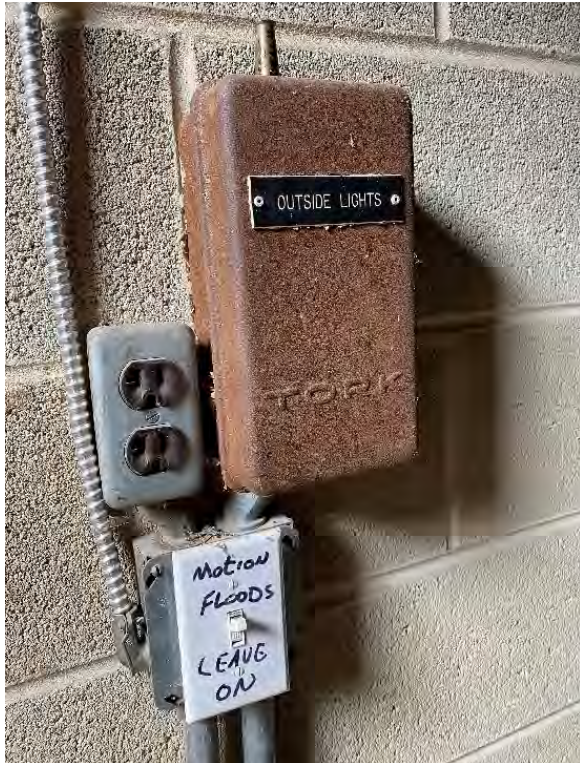
Time Clock / Unprotected Receptacle
