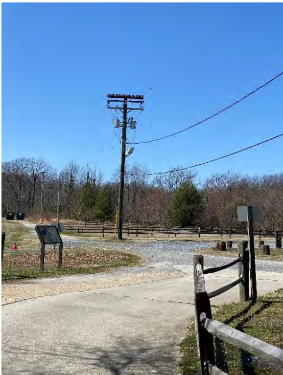
Pole-Mounted Utility Transformers
