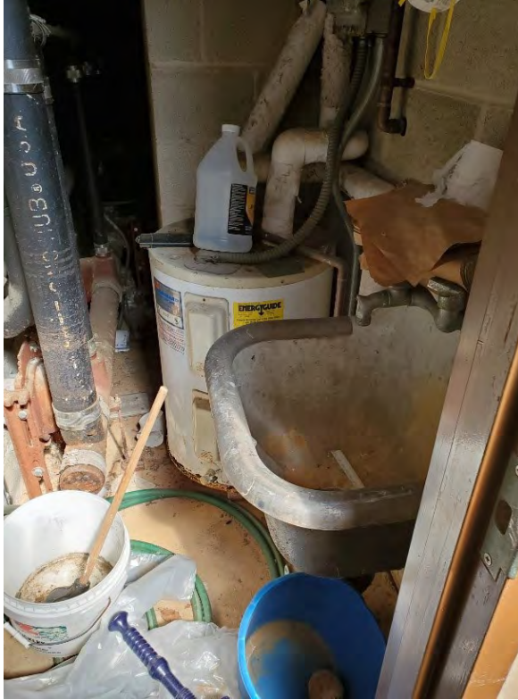
Janitor Closet Sink
