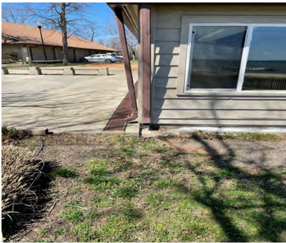
8.4.1 Example of downspout discharge.
