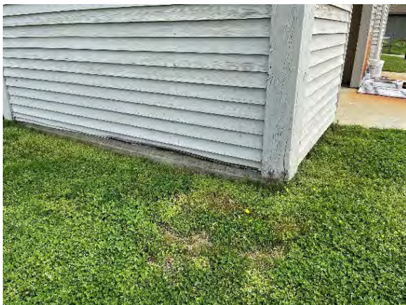
Exterior Elevation -Note the damage to the siding.
