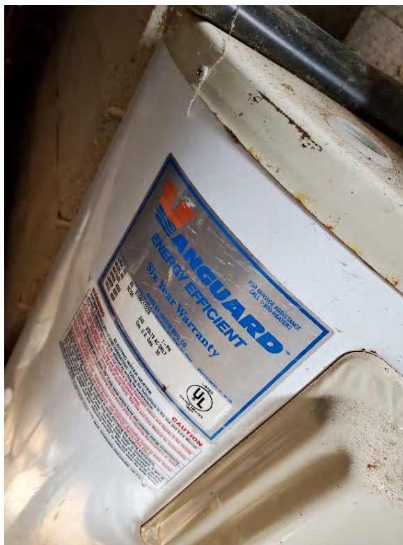
Domestic Water Heater
