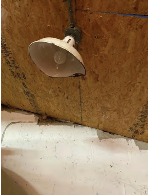
Interior Light not Working
