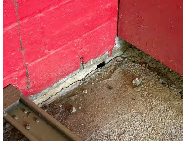
View of settled floor slab in the storage area.
