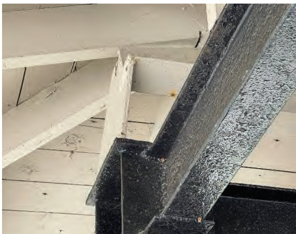
Interior view of roof beam connection by a gusset plate. Recommend enhancing this connection.
