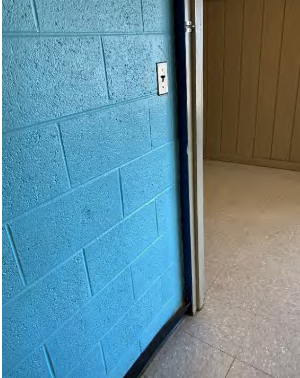
Typical Restroom Switch
