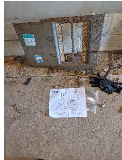
Dead front below panel.
