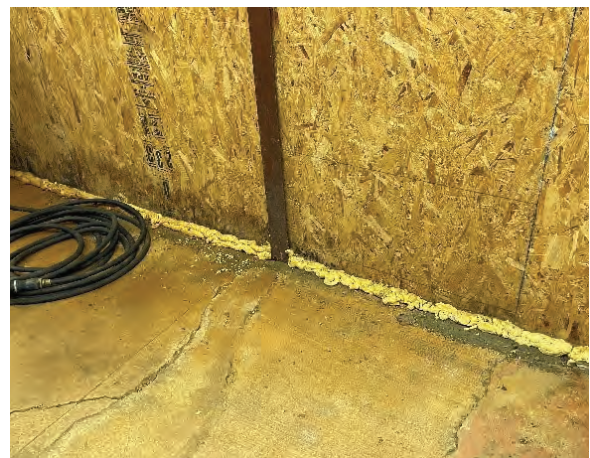
Spray foam sealing of wall base. Note floor cracking.
