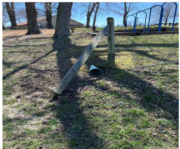
8.4.4 Pipe discharge with no outfall protection.
