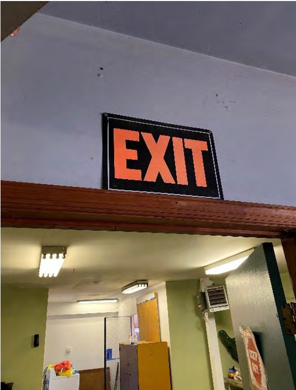
Room 401 - Non-Illuminated Exit Sign
