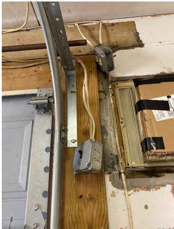
Hanging Receptacle and Switch
