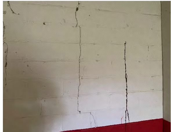
Minor vertical cracking distress in work zone wall.
