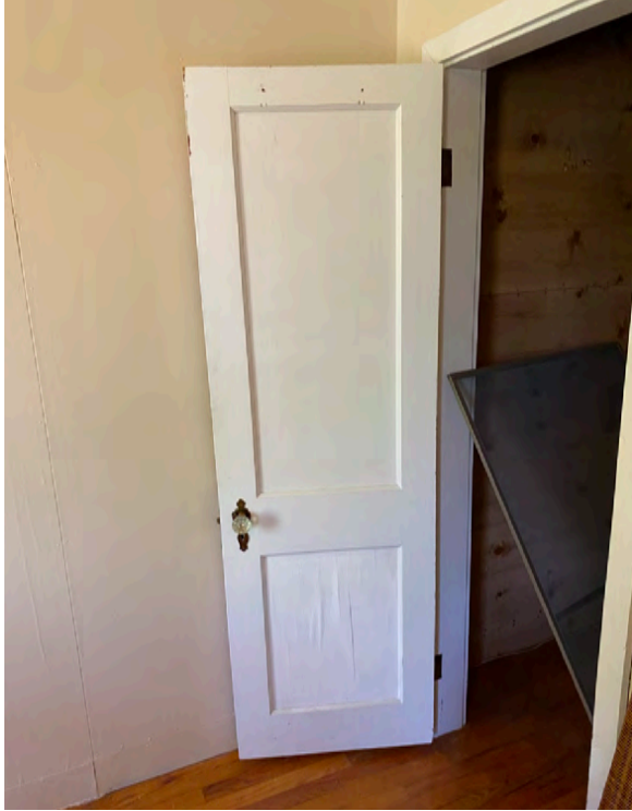
Lower panel damage at 210/B
