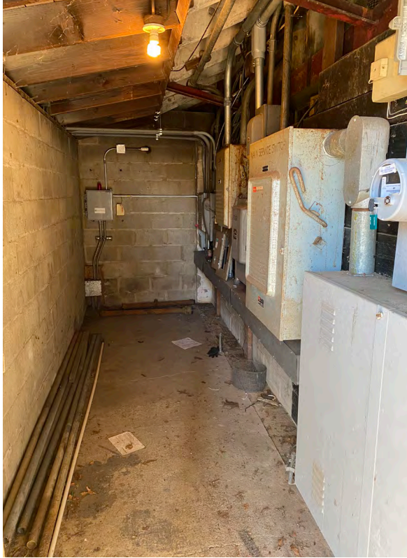
Room 411 - Electrical Room
