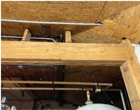
View of distressed lintel in enclosed portion.
