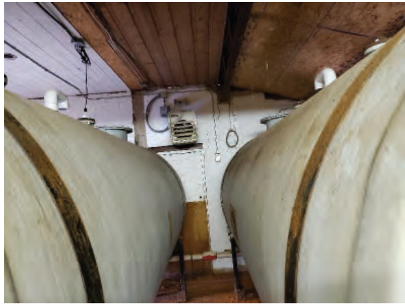
Well Booster Pump Storage Tank
