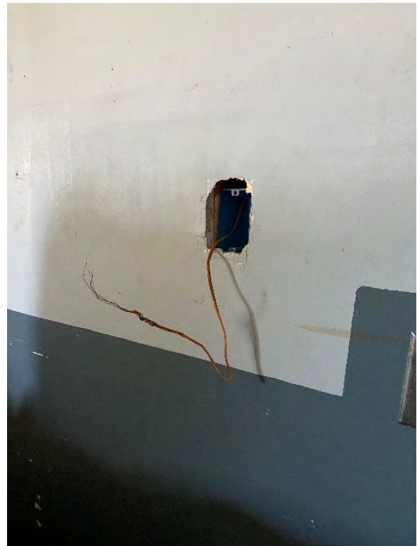
Abandoned Cabling (Typical)
