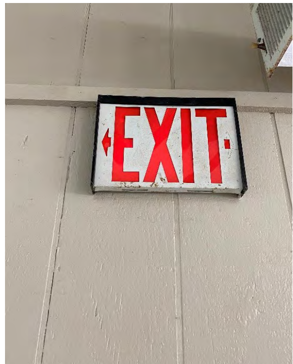
Damaged/Non-illuminated Exit Sign
