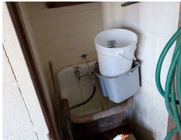
Janitor Closet Sink
