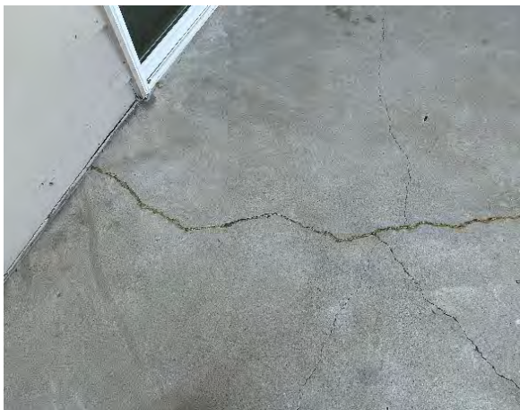
Exterior slab shrinkage cracking
