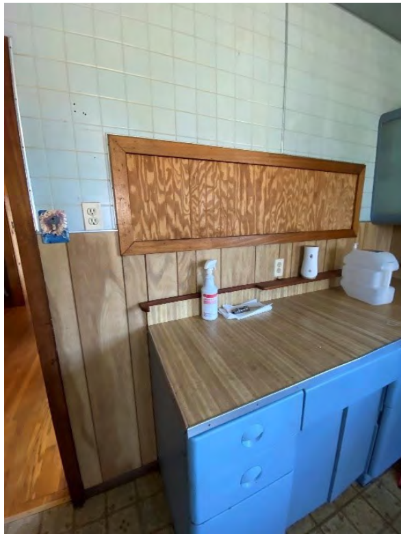
Kitchen Countertop Receptacle
