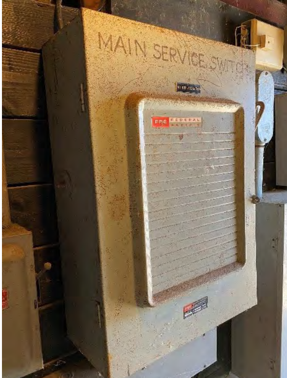
Room 411 - Main Service Disconnect
