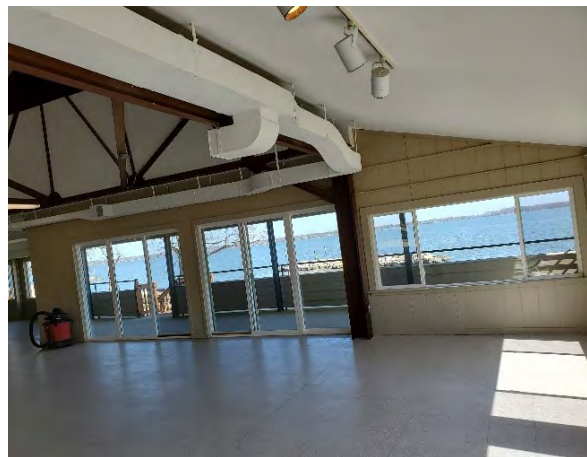
Common Area Ductwork
