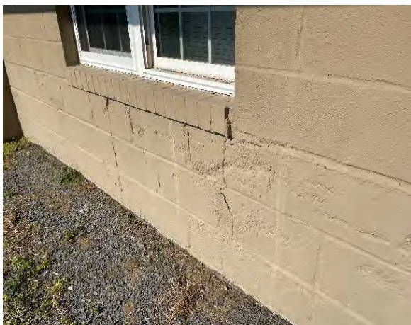
Exterior masonry area where surface pitting is visible.
