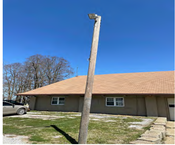
8.6.2 Existing spotlights on wooden pole
