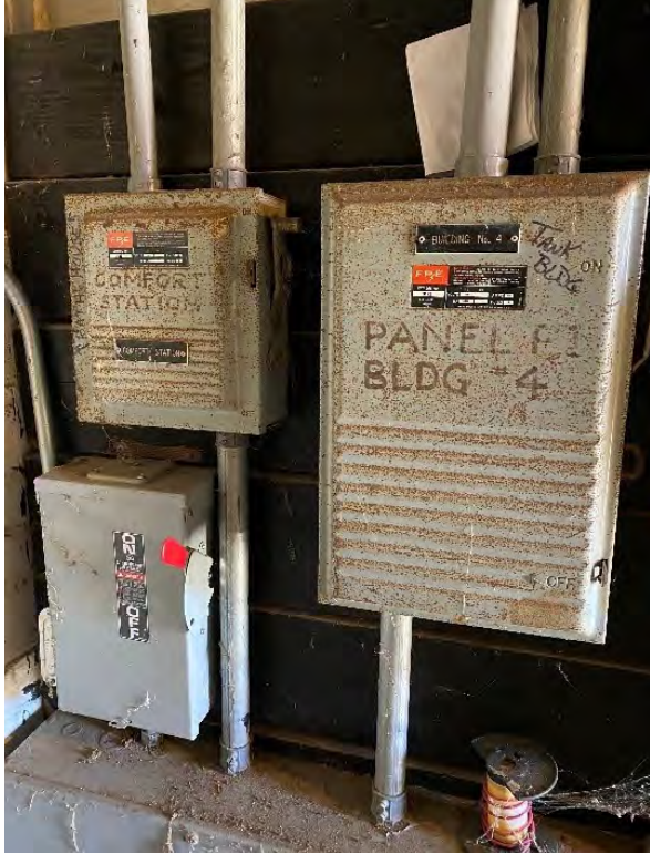
Room 411 - Typical Disconnects
