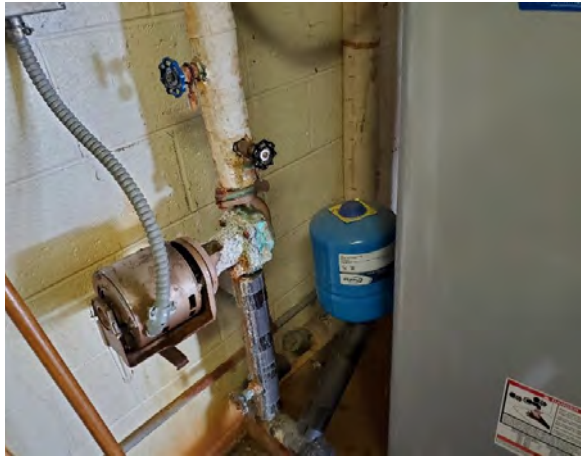
Expansion Tank and Recirculating Pump
