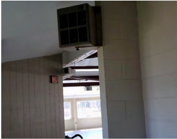
Corridor Unit Heater
