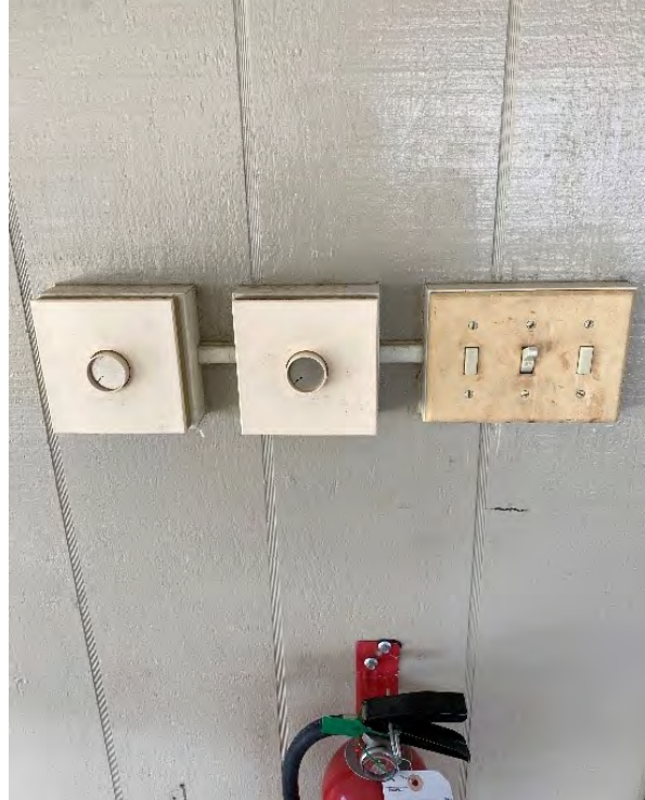
Outdated Dimmer Switches
