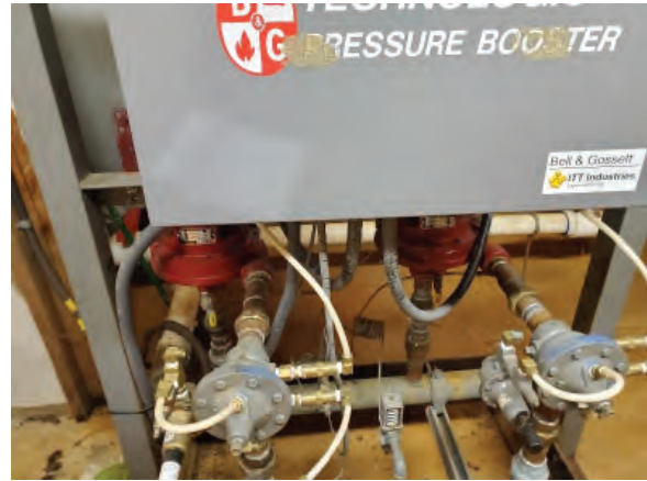
Well Booster Pump
