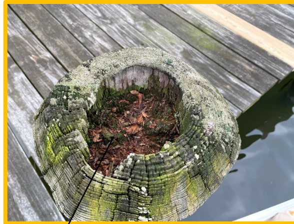
Necking and Pitting of Piles
