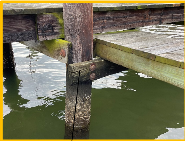
Splitting of Support Members
