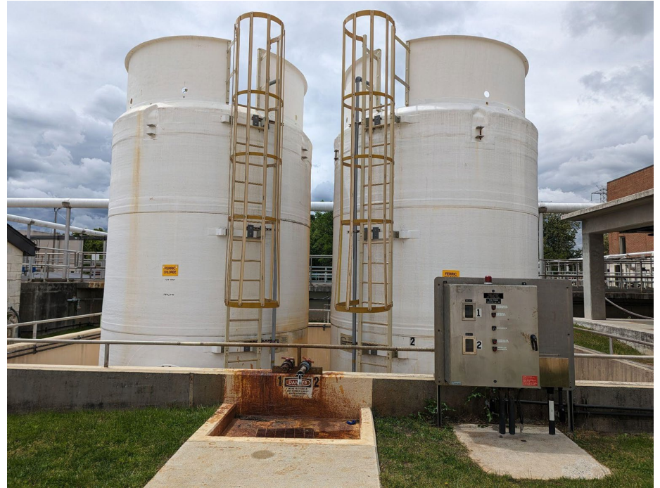
Ferric Chloride Tanks, Cox Creek WRF
