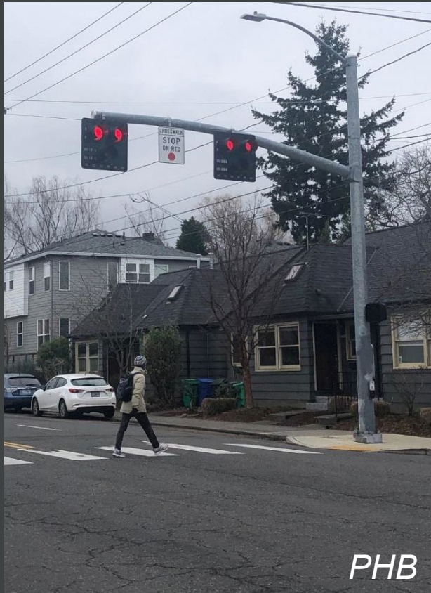
Rapid flashing beacon
