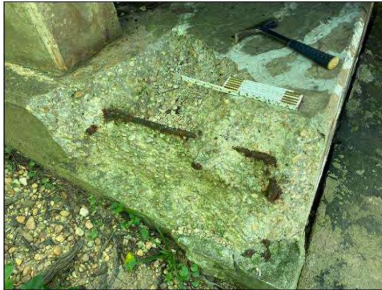
Photo 18 - Spall with Exposed Corroded Reinforcement at West End of North Abutment
