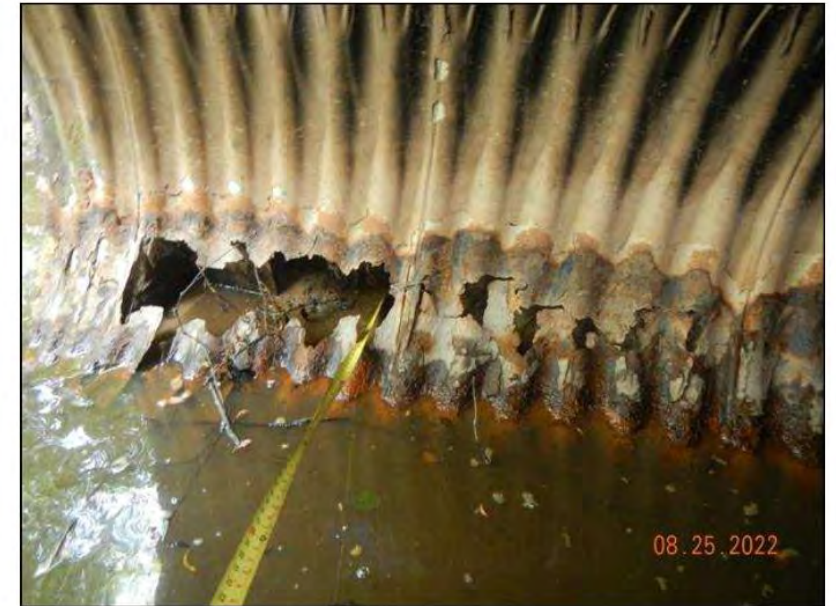
Photo 16 - Area of Section Loss in Pipe 2 in West side of South End
