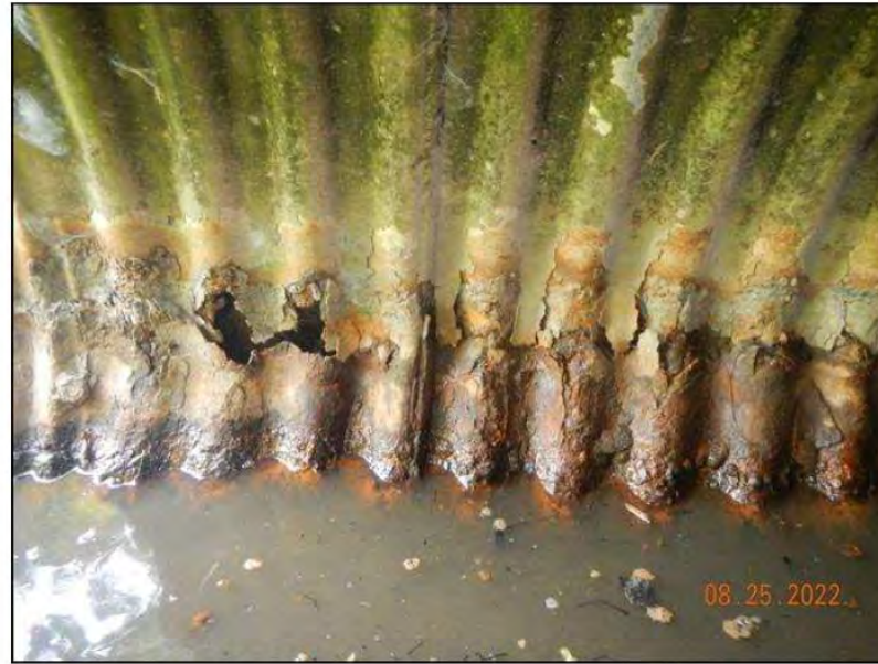
Photo 12 - Area of Section Loss in Pipe 1 on West Side of South End
