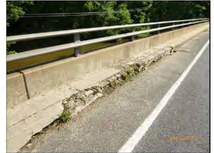
Photo 9 - Spalling with Exposed Corroded Reinforcement in West Safety Curb at Mid-Span of Span 2
