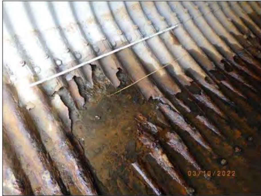
Photo 10 - Area of 100% Section Loss in the North Side of the Invert at the Upstream End of Cell 1 (Approximately 5ft into the Cell Shown)
