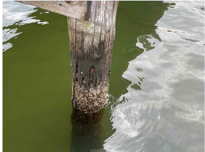
Photo 6 – Piling necking at the waterline
