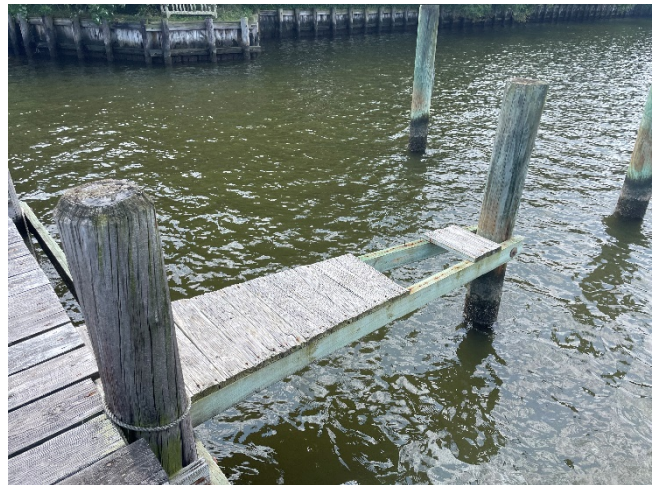
Photo 8 – Missing Decking Boards
