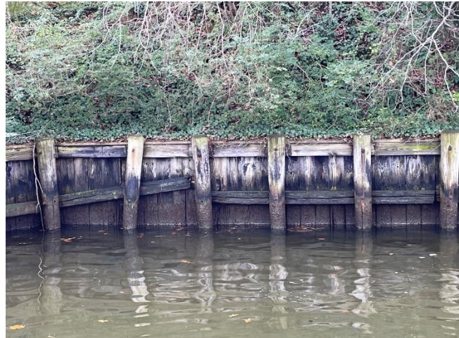
Photo 2 – Deteriorating bulkhead members
