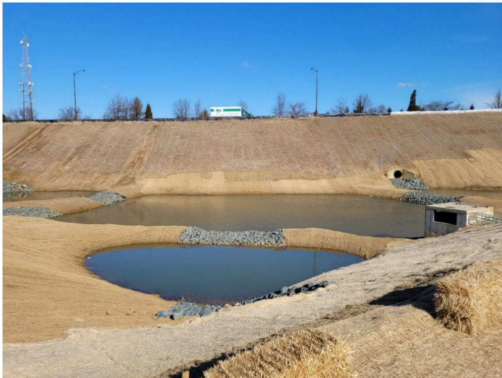
Figure 3-4: MD 665 Stormwater Management Facility, Facing Northeast
