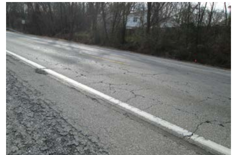
Typical pavement condition
