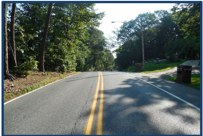
PHOTO 2: INSUFFICIENT SIGHT DISTANCE AT VC- 3
