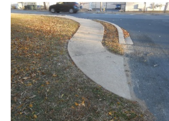
Figure 46 - Existing Pedestrian Ramp just south of SW Corner of Odenton Road Intersection
