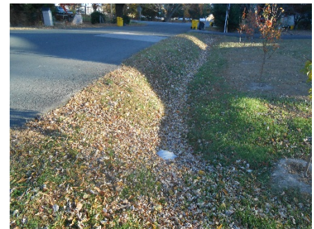
Figure 41 - 495 Greenwood Street - Drainage Ditch
