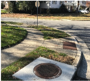
Figure 1 - Existing Pedestrian Ramp West Side of Hillcrest Road at Maple Ridge Lane
