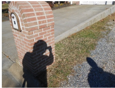
Figure 26 - Existing 1194 Monie Road Driveway Retaining Wall/Curb - Needs to be Reconstructed
