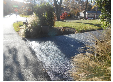
Figure 30 - South Side of Hammond Lane Looking South - Steep Roadside Grading / Landscape Removal
