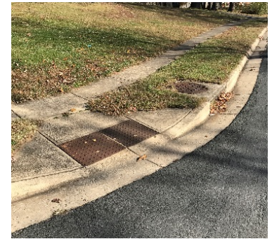
Figure 3 - Existing Pedestrian Ramp East Side of Hillcrest Road at Maple Ridge Lane
