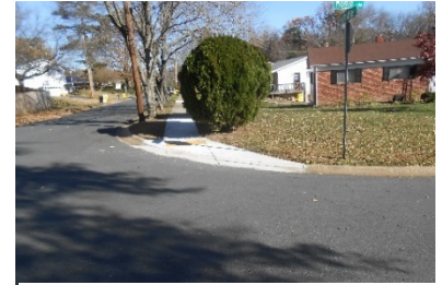
Figure 24 - NE Corner of Maple Ridge Lane Intersection - Existing Pedestrian Ramp / Shrub to be removed
