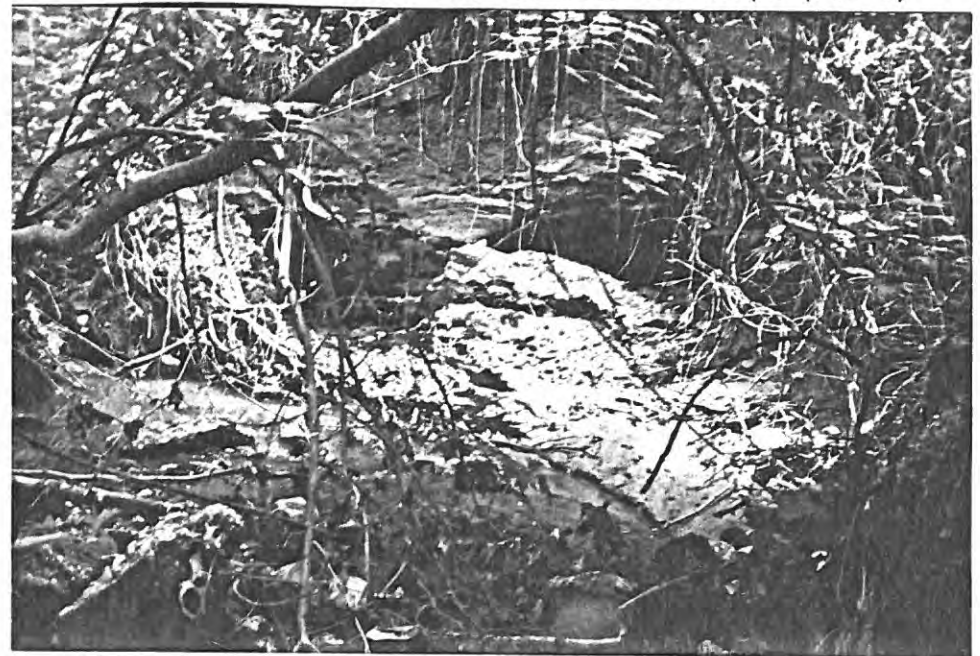
Photo 4 Undercutting of Steep Banks on Weems Creek at U.S. Rte. 50 and MD. Rte. 450 Ramps (Pt. D)
