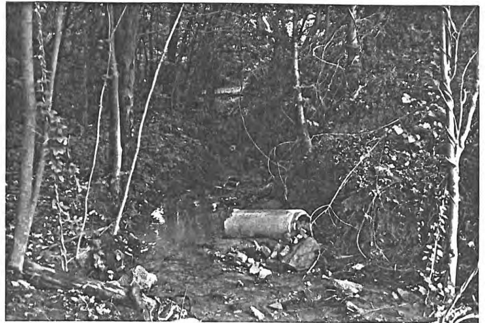
Photo 8 Bank Sloughing and Erosion on Weems Creek (Pt. H)
