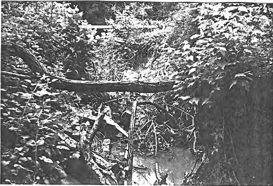
Photo 7 Bank Erosion Undercutting Trees on Weems Creek (Pt. G)
