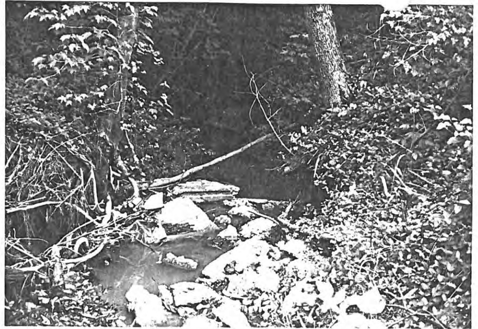
Photo 6 Channel Degradation and Bank Failure on Weems Creek (Pt. F)
