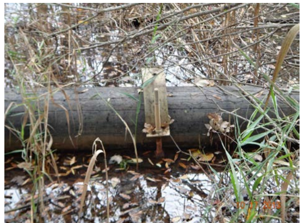
Exposed Utility in the Parrish Creek Subwatershed (WRA) with Moderate Impact Score
