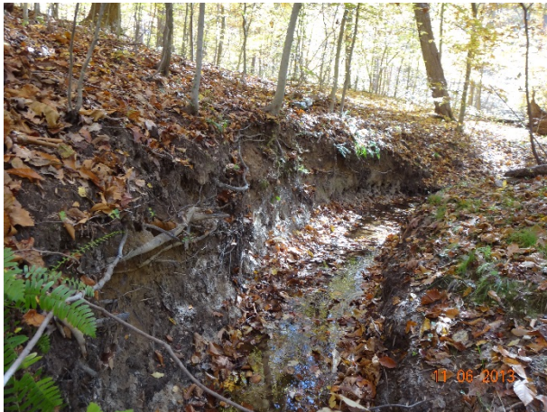
Bank Erosion in the South Fork Muddy Creek II Subwatershed (RR5) with Moderate Impact Score
