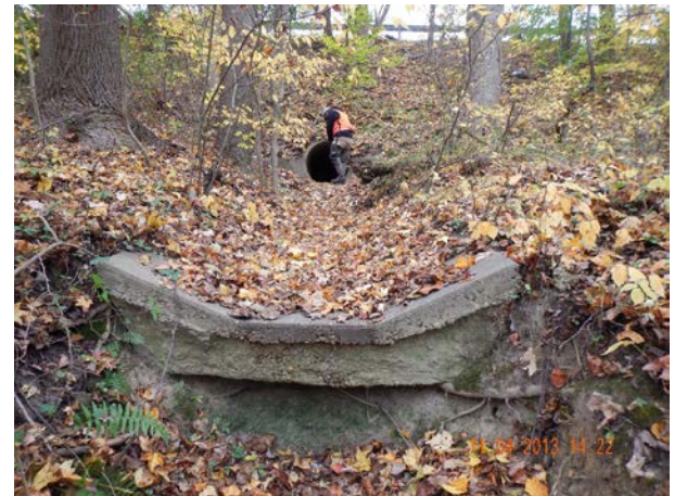
Outfall in the Many Fork Branch Subwatershed (RR3) with Moderate Impact Score
