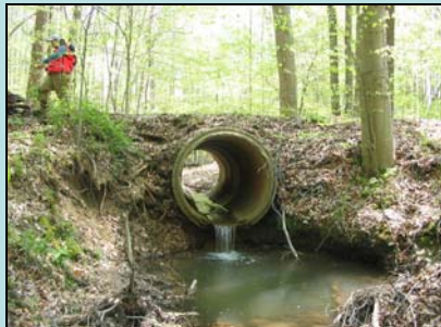
Crossing with severe impact score located south of Harwood Rd.
