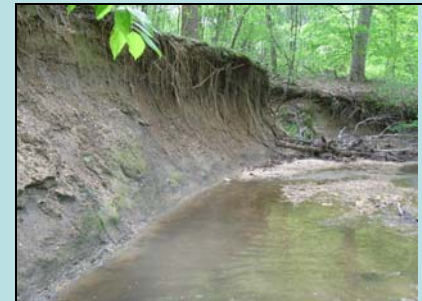
Erosion with severe impact score on stream between Harwood Rd. and Queen Anne Brige Rd.
