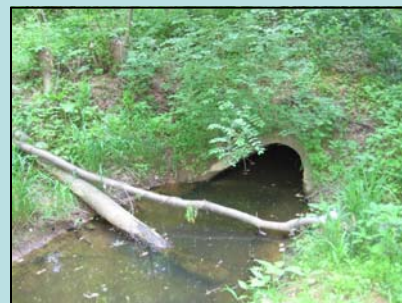
Ditch with minor impact score located near Brock Bridge Road outside of Laurel
