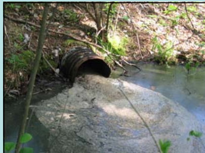
Crossing with severe impact score located in Patuxent Research Refuge
