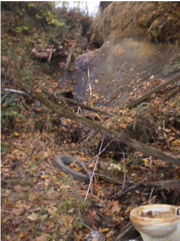
Photo 6. Impaired Reach. View large headcut and debris looking upstream
