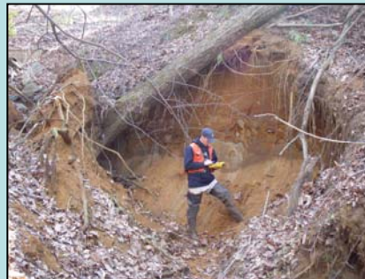
Erosion with extreme impact score located just south of Defense Highway.
