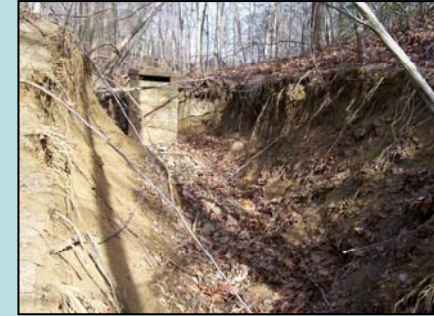
Pipe/Ditch with severe impact score located off Cinnamon Lane.
