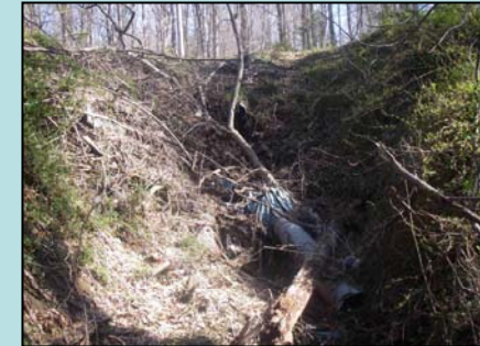
Pipe/Ditch with severe impact score located just south of Mount Tabor Road.
