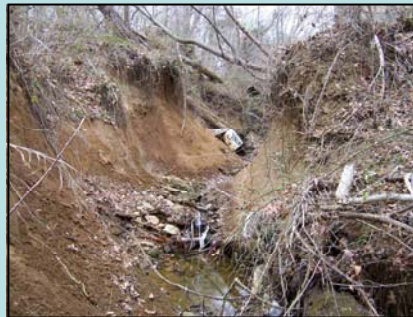
Erosion with extreme impact score located near Riva Road in the vicinity of Riva Dr.
