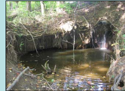
Pipe/Ditch with severe impact score located near the end of Aisquith Farm Road.
