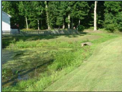
Deficient Buffer with extreme impact score located near North Carolina Avenue.
