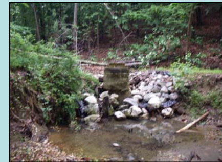
Utility with extreme impact score located next to Shady-water Way.
