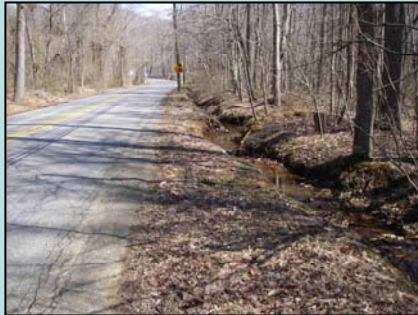
Deficient Buffer with extreme impact score located east of Rutland Road.
