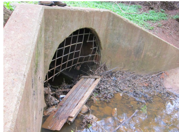
Photo 12 – Inlet where both stream reaches return to piped flow
