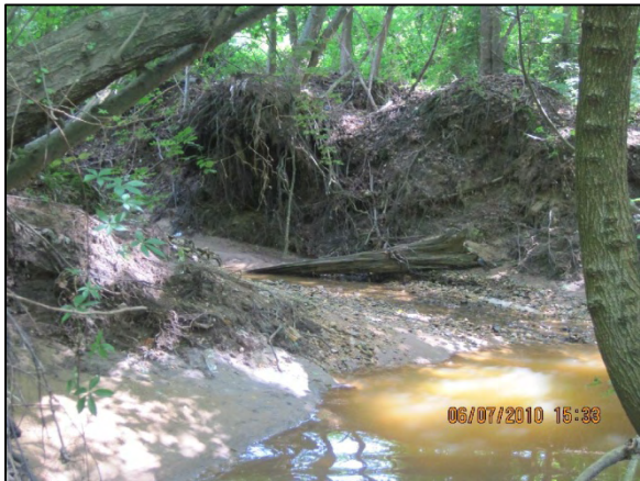
Photo 9 – Severe Bank Erosion
