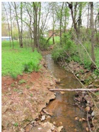
Photo 5 – Cement armoring currently along downstream portion of Reach 2
