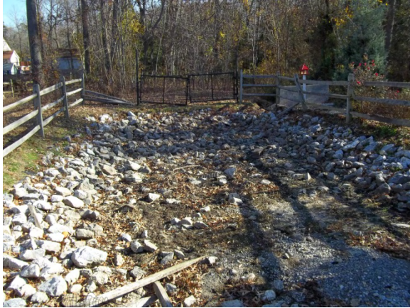
Photo 1 – Existing infiltration BMP at end of 209 th Street in dry condition (looking downstream)
