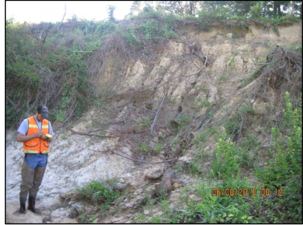
Photo 8 – Extreme Bank Erosion Downstream of Culvert
