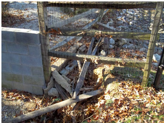
Photo 3 – Inadvertent spillway for existing infiltration BMP
