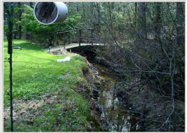
Downstream from Mid-Point
