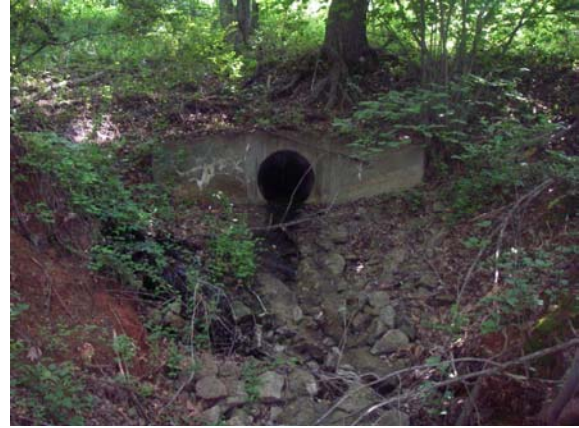
Pipe and ditch impacts contributing to erosion. Moderate Impact in the Stoney Run 1 Subwatershed (PN6)
