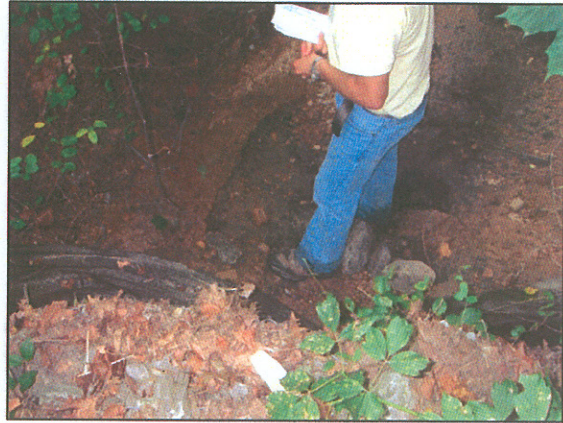
PHOTO 2: VIEW OF SCOUR HOLE FROM TOP OF HEADCUT
