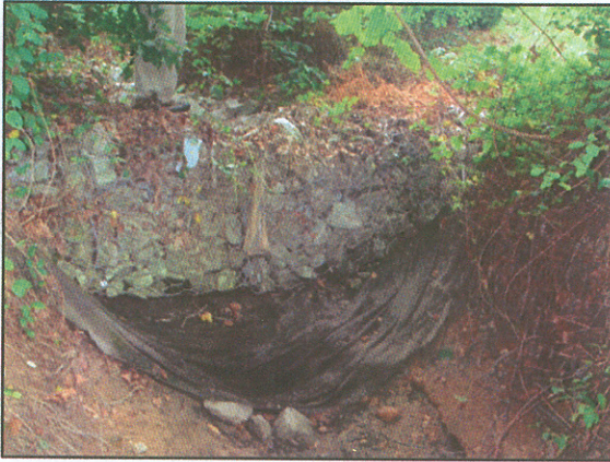
PHOTO 1: FAILING GABION BASKET FACING UPSTREAM
