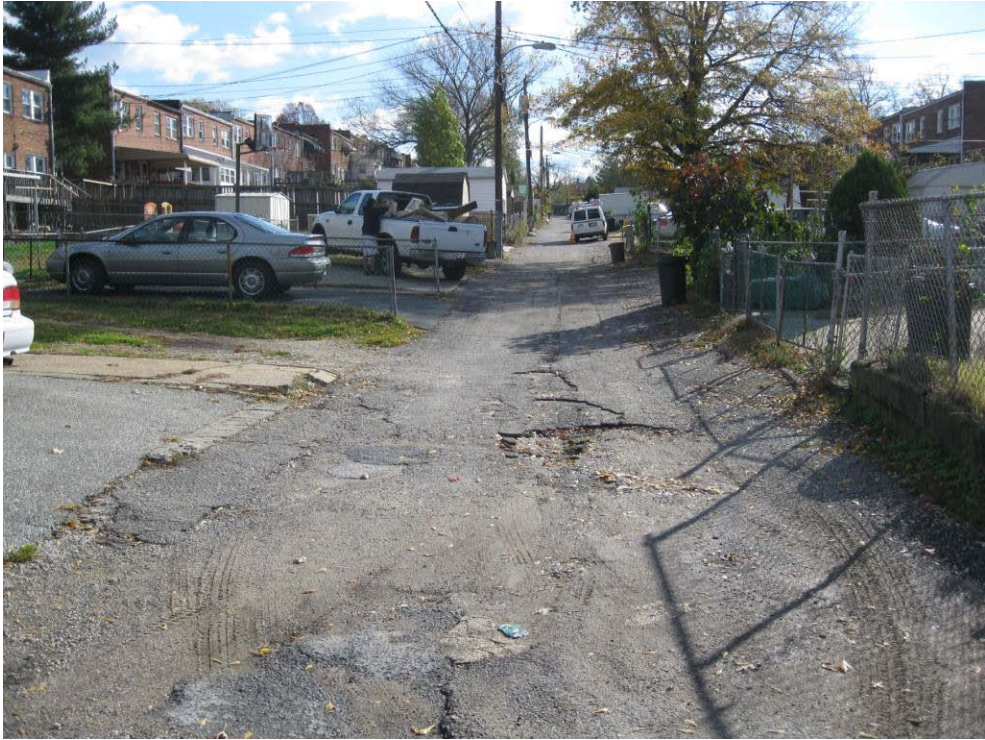
PHOTO 1: EXISTING ALLEY WAY (NOTE THE POOR PAVEMENT CONDITION)
