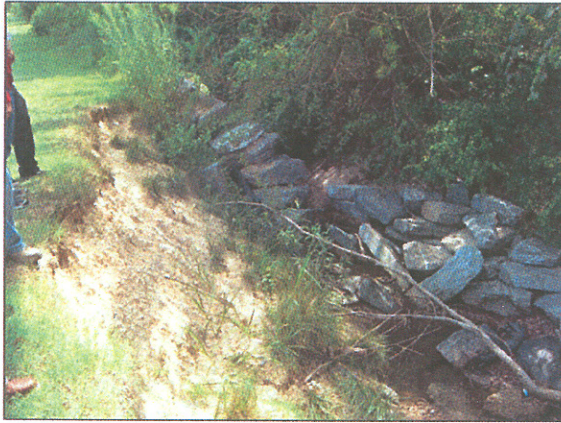
PHOTO 1: VIEW OF FAILING IMBRICATED WALL
