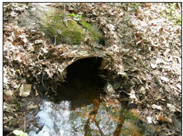
Stream Crossing with Moderate Impact in the Deep Creek Subwatershed (MGT)
