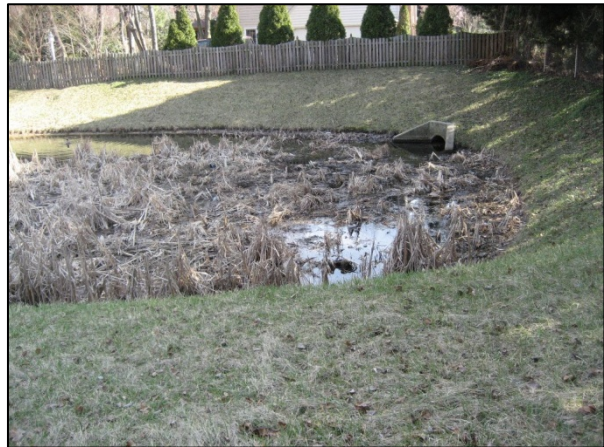
Poorly Performing Infiltration Basin near Dunkeld Court in the Cypress Creek Subwatershed (MGC)
