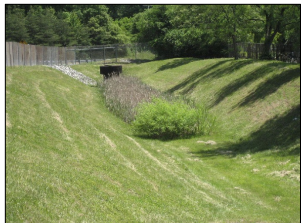
Poorly Performing Extended Detention Pond near Leelyn Drive in the Cypress Creek Subwatershed (MGC)
