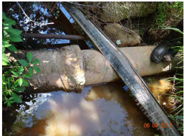
Exposed Utility in the Little Patuxent 2 Subwatershed (LP0) with Moderate Impact Score
