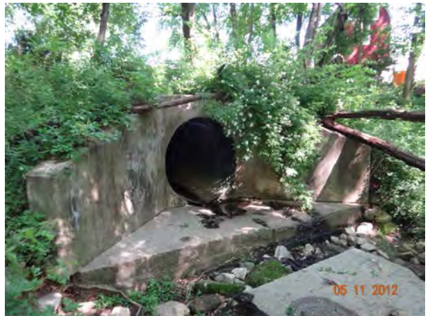
Outfall in the Towsers Branch 1 Subwatershed (LP3) with Moderate Impact Score
