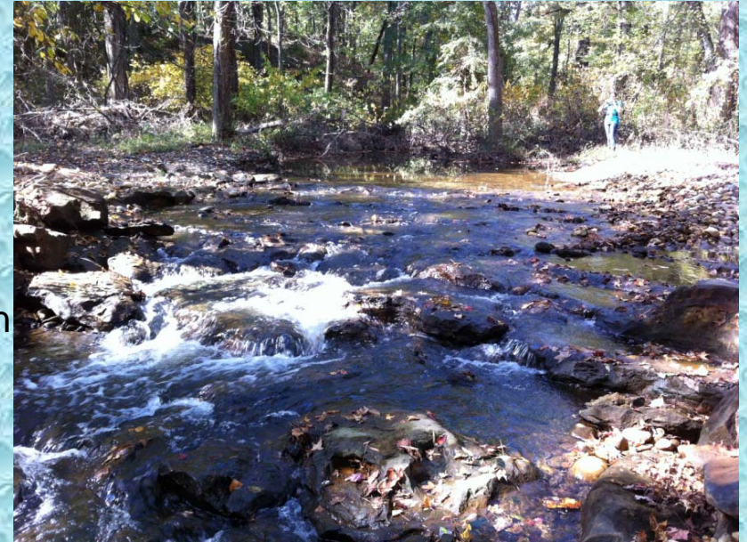
Severn Run Mainstem, 3 feet high 30 ft long in-stream weir was used to connect 150 feet of stream to the floodplain.
