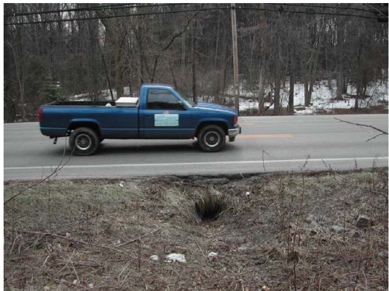
Existing culvert under Mountain Road near Loblolly Lane is too small for all but the smallest mammal species
