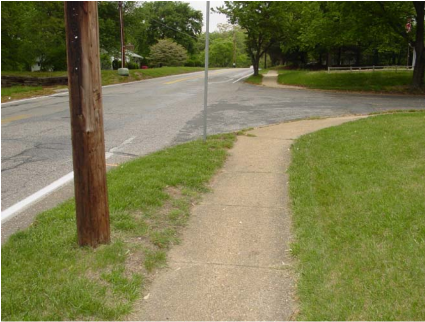
EXISTING DETERIORATED CONCRETE SIDEWALK AT INTERSECTION OF PASADENA ROAD AND BROOKVIEW AVENUE
