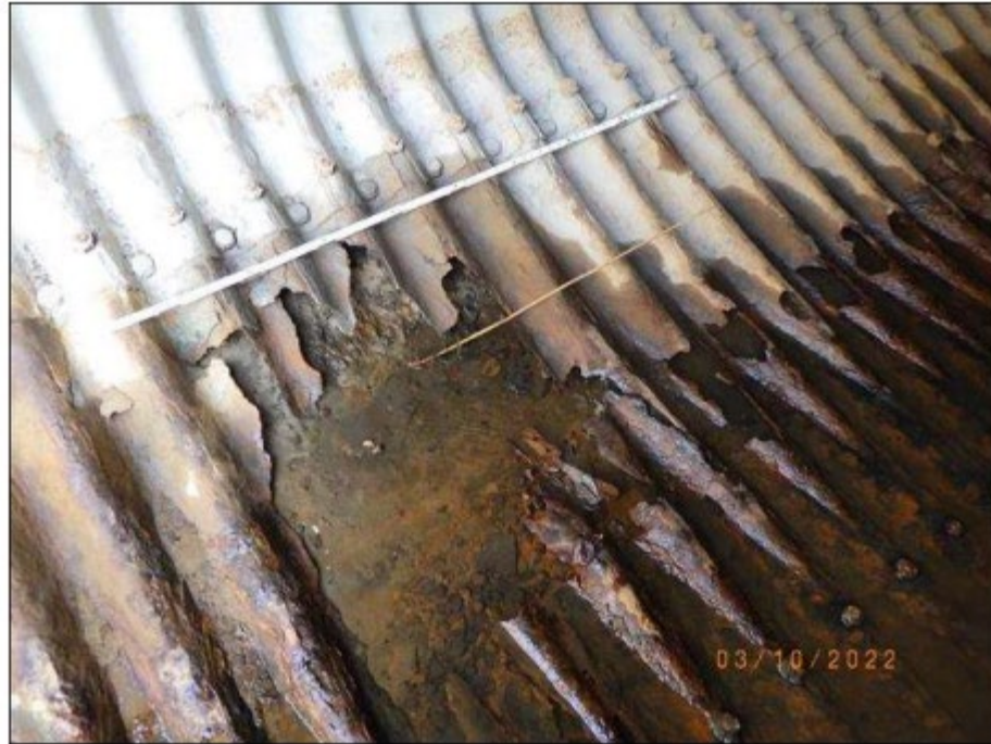
Photo 10 - Area of 100% Section Loss in the North Side of the Invert at the Upstream End of Cell 1 (Approximately 5ft into the Cell Shown)
