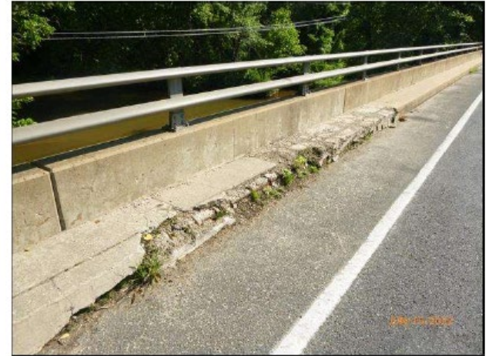
Photo 9 - Spalling with Exposed Corroded Reinforcement in West Safety Curb at Mid-Span of Span 2
