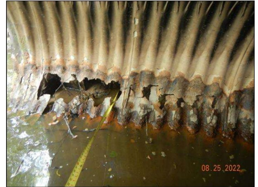
Photo 16 - Area of Section Loss in Pipe 2 in West side of South End
