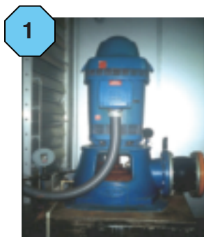
1 Wells (well pump at a water treatment facility)
