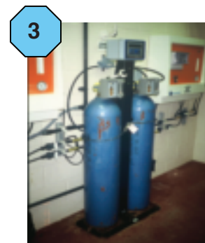
3 Chemical Addition (chlorine feeders)
