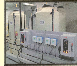
Chemical Feed Pumps
